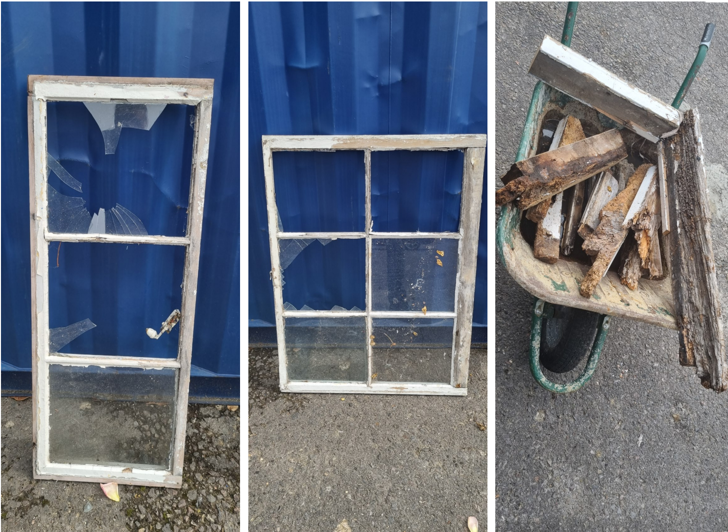
Photos 7-9: Photographs of the surviving fabric of the rotten windows that were re removed illustrating that the frames were beyond repair and in need of full replacement. These were inspected by the Council's Conservation Officer in September 2022 pursuant to a pre-application enquiry process (Ref: 2022/1555/L2PA).
