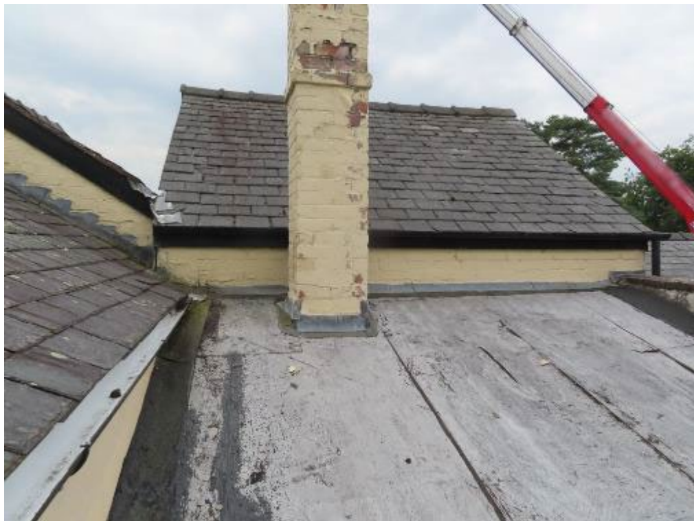
Photograph 4. Exterior. Lower left: part of the Section 4 Southwest elevation roof-slope. Upper left: part of the Section 5 Northwest elevation gable. Lower centre and right: part of the Section 2 roof structure. Upper centre and right: Northwest elevation of Section 6.
