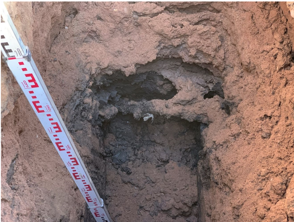
Photograph 35: TP11. Potential service. Sample taken from unknown material, laboratory testing confirmed material to be weathered wood..
