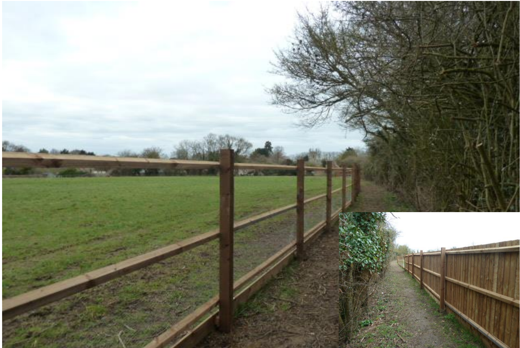
IMAGE 32 – Another view through the yet to be completed paddock fence on its eastern side (lying outside of the site), looking north. It shows the ‘retained’ paddock area. The fence has created an enclosed corridor for a footpath linking Church Lane to Cornells Lane. Views from this will be curtailed once fencing is completed as allowed under permitted development rights. The inset photograph shows that views towards the application site from beyond the north–east side of the paddock are curtailed by the completed fencing.
