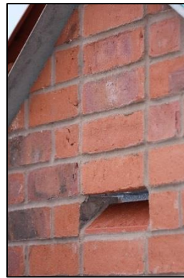
Figure 2: Habibat Bat Box faced with red brick, incorporated within wall at gable end.
