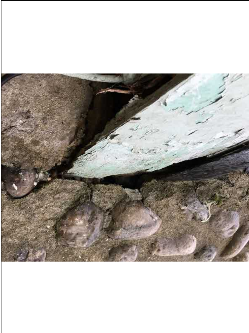
Photo 9. Potential roost feature between soffit and chimney. The crevice contained <10 potential bat droppings
