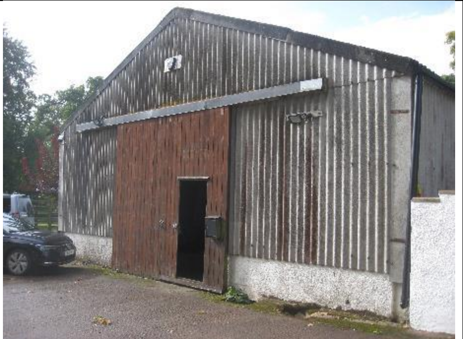
Photo 1: Building B1 showing the side panels and wooden doors of the east elevation.
