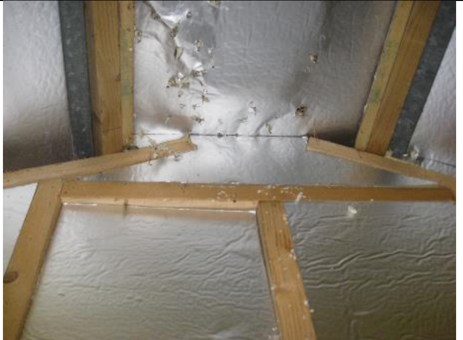
Photo 7: Building B1- insulation in roof of storage area damaged by squirrels.
