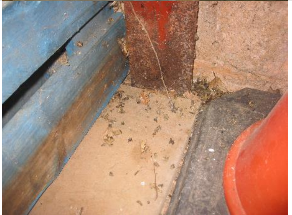
Photo 8: Building B1- mice droppings found at the bottom of metal supporting post at the east end of the building.
