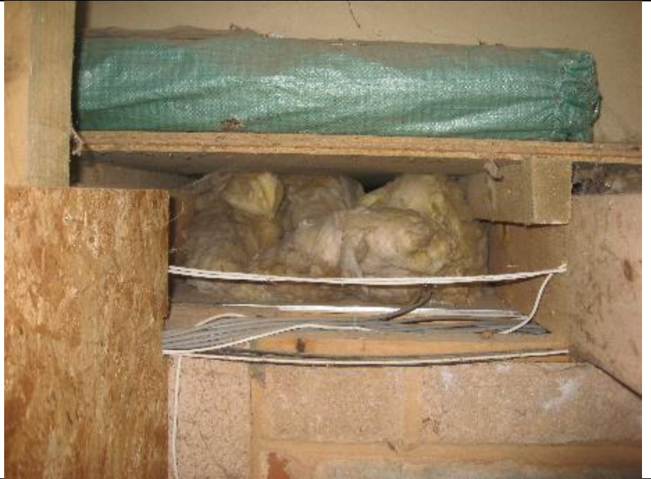
Photo 5: Insulation above the office and below the storage area that is above the office.
