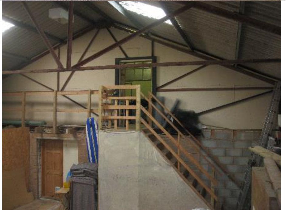
Photo 2: Building B1 interior open storage space with door to office below and more insulated storage space above.
