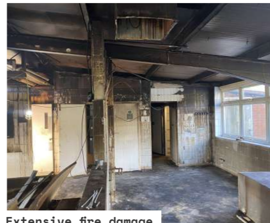
Extensive fire damage
