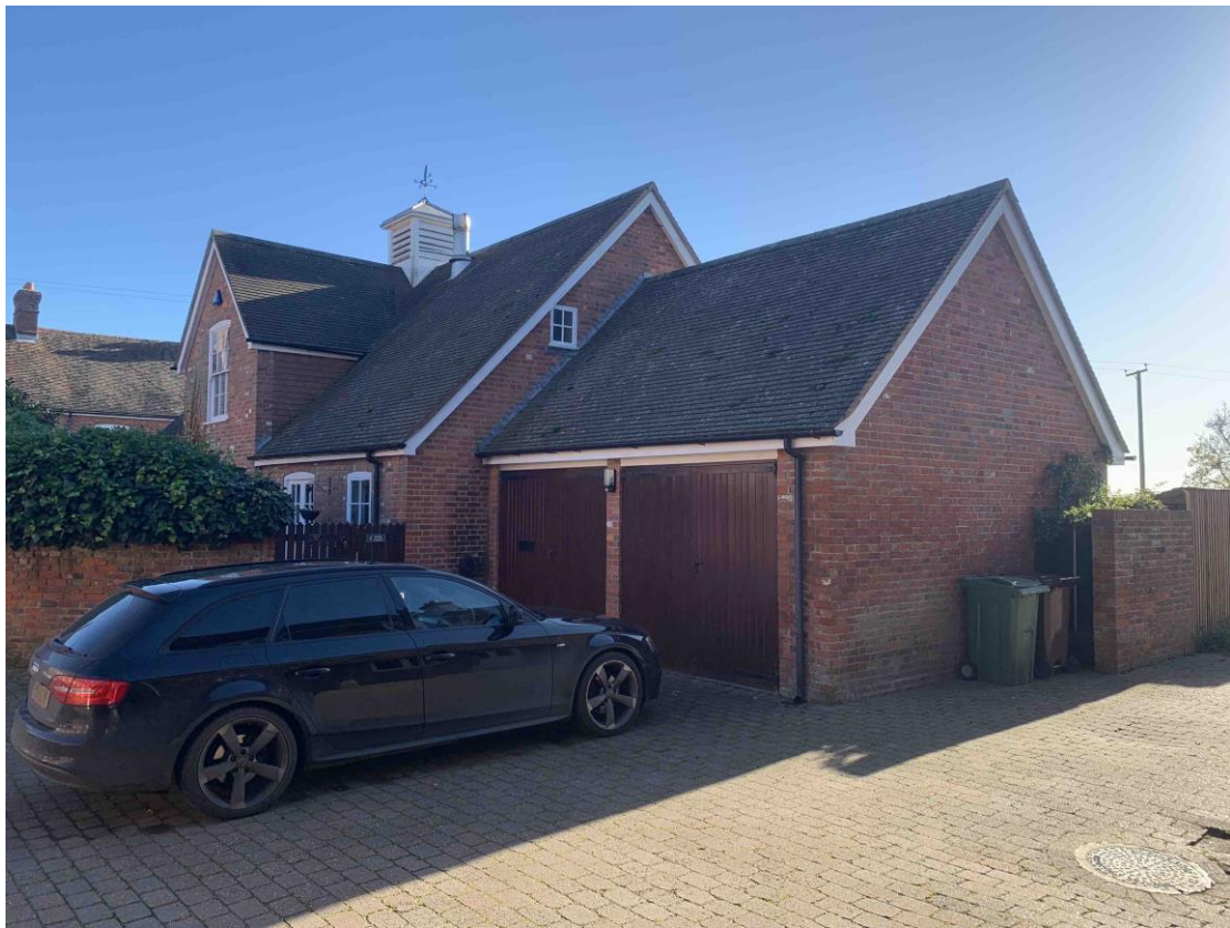
Front of the house from the western end of the courtyardRotten back bedroom window
