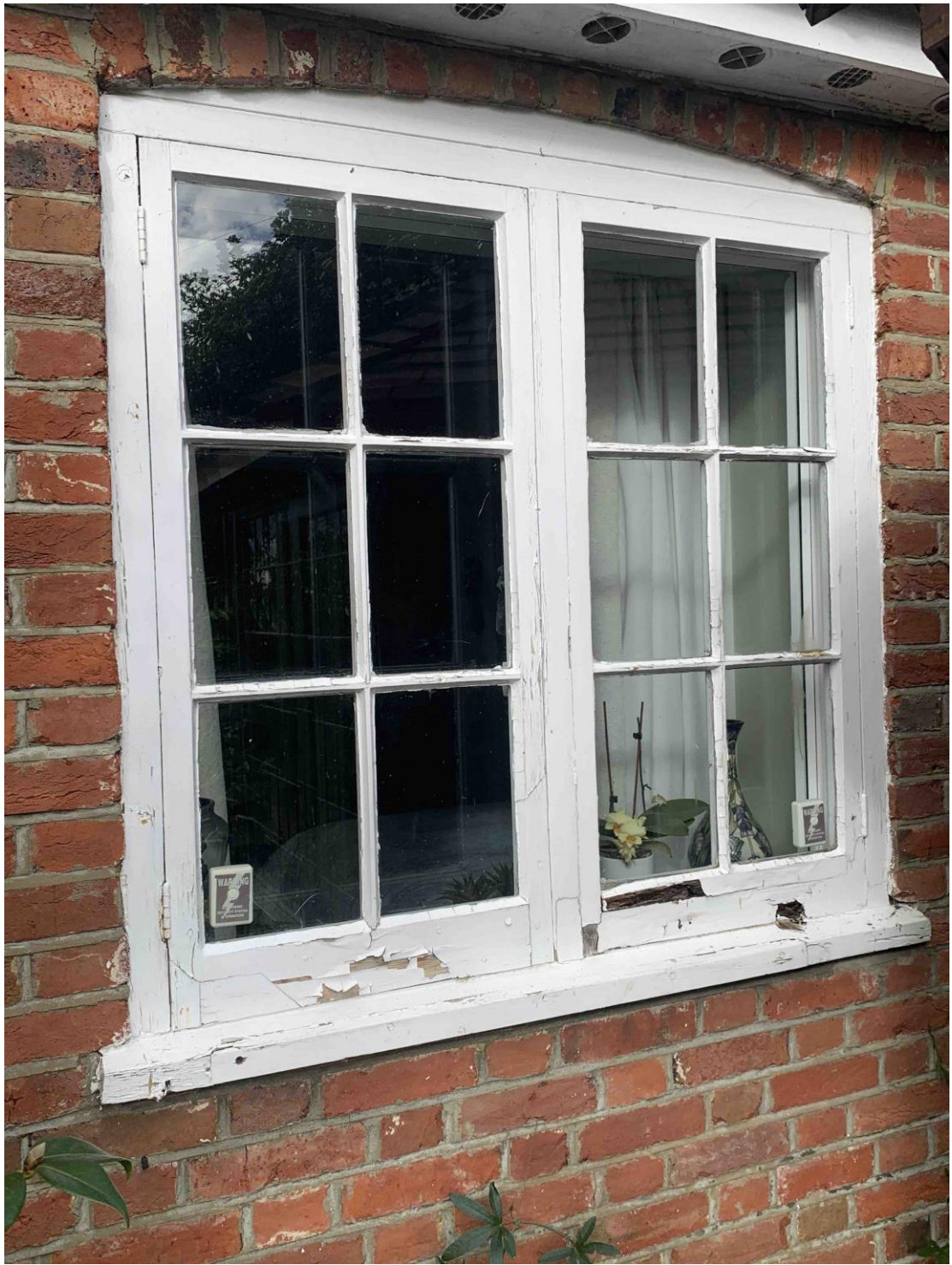
Rotten Back window to be replaced with doors from the kitchen
