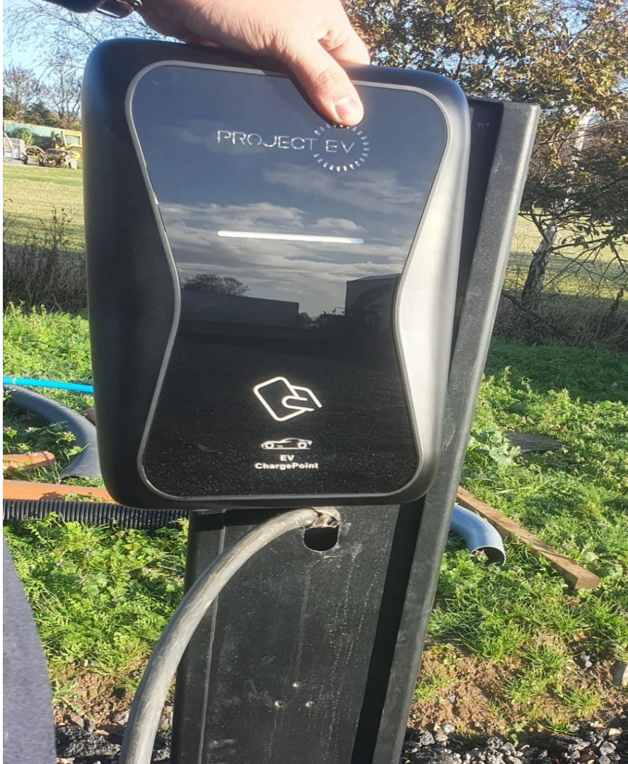
Figure 2 Example of Charger unit
