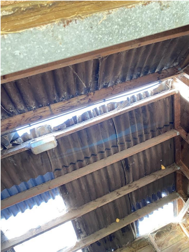
Plate 10 – Gaps in roofing
