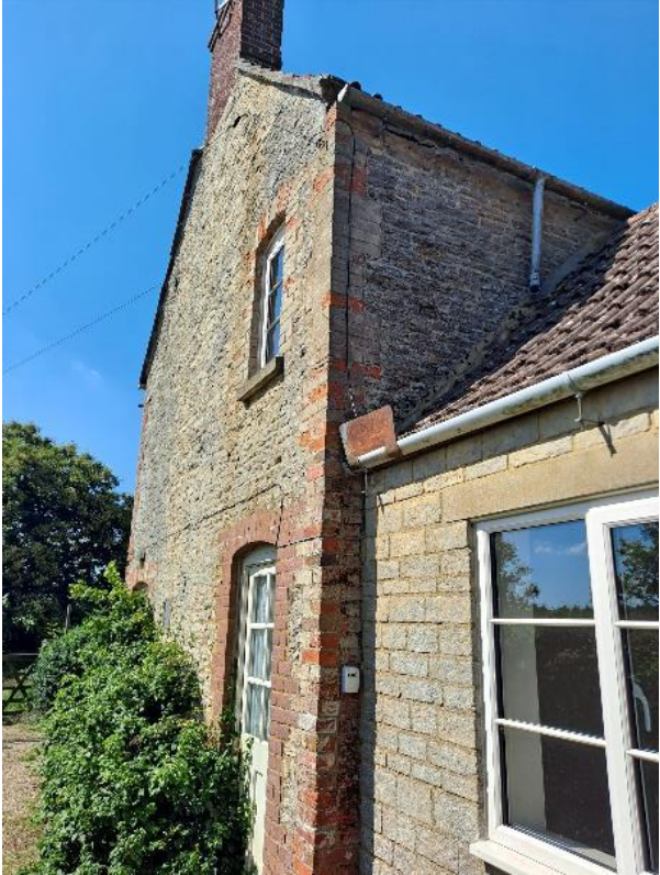
Photograph 7. The east elevation of Colly Lodge, the location of gaps at the roofline (Target Note 7).
