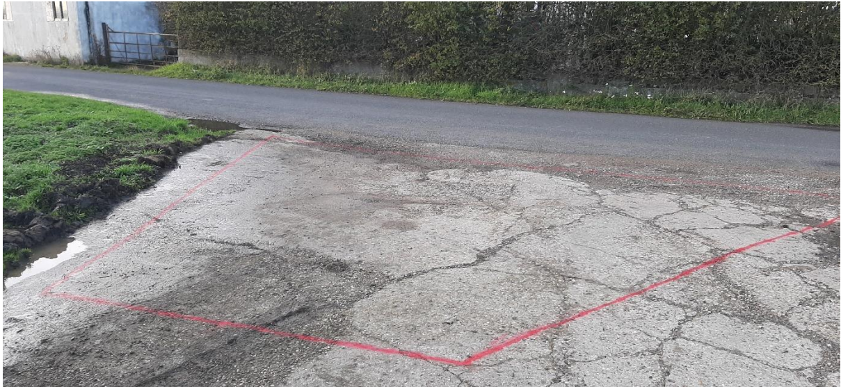
Figure 1 Existing access area sloping away from the highway
