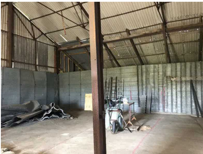
Figure 4: October 2022 -Internal view of north-west corner, where broken asbestos roof has now been replaced.
