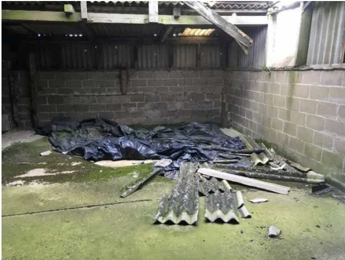
Figure 3: May 2020 - Internal view in north-west corner of the barn, where asbestos roofing had degraded and fallen in.
