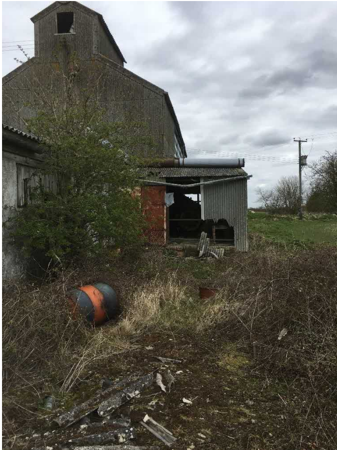
Figure 5: 2020 - View looking east across the back of the barn. Overgrown with vegetation and broken asbestos sheeting, and metal drum.
