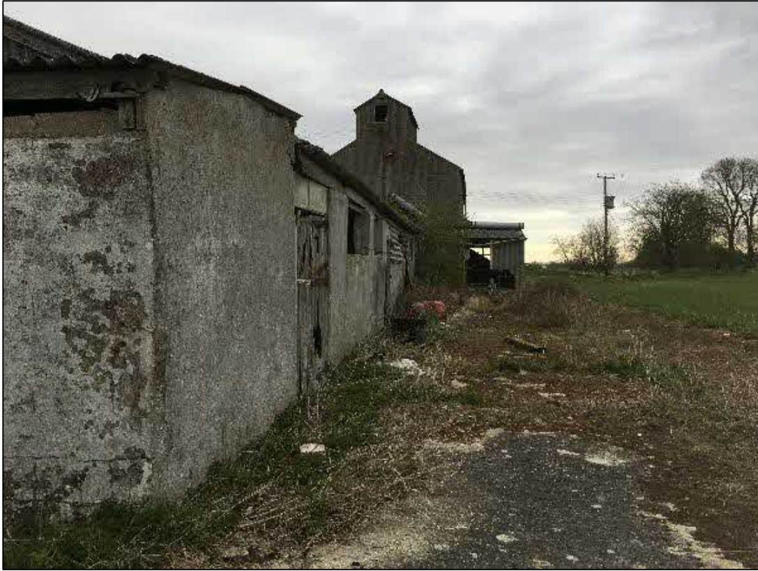
Concrete Apron to South of Main Structure with Visible ACM Fragments on Surface
