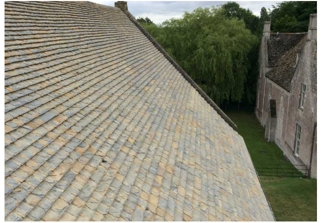
Slate tile hanging and new extensions roofs to be faux Collyweston as shown.
