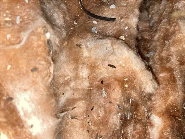
Bat dropping in north section of farmhouse roof space
