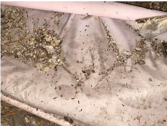
Bat droppings in south section of farmhouse roof space
