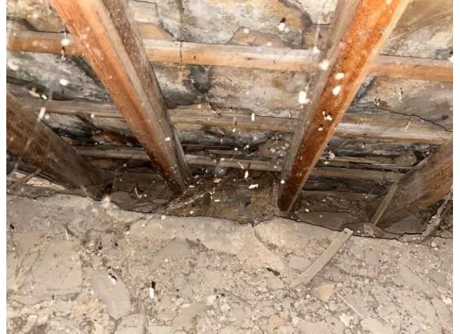
Bird nest in south section of farmhouse roof space
