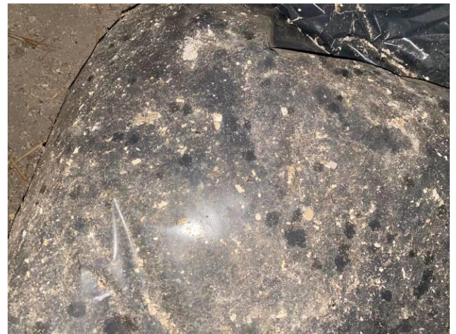
Urine stains in south section of farmhouse roof space
