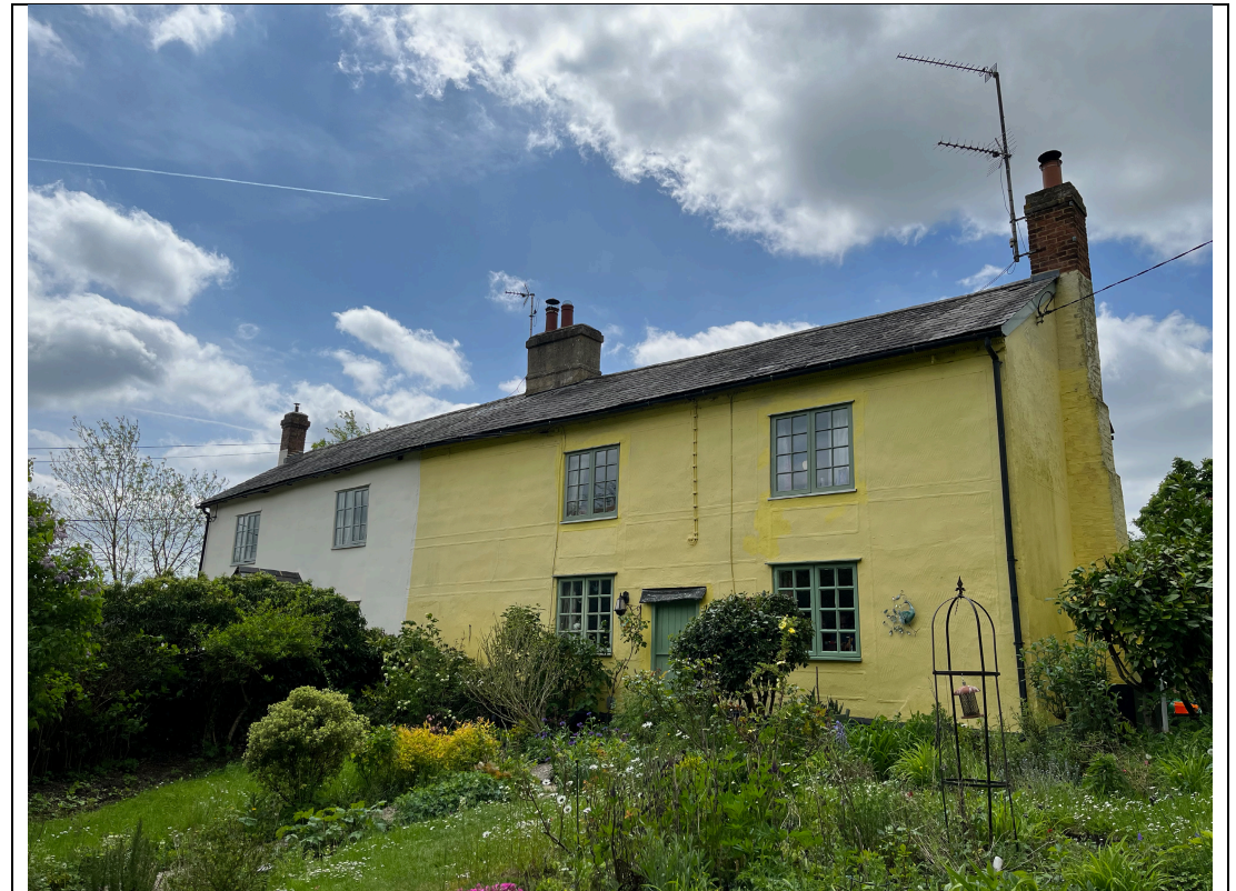
The front of 2 Lower Farm Cottages with its render fielded panels with feathering.
