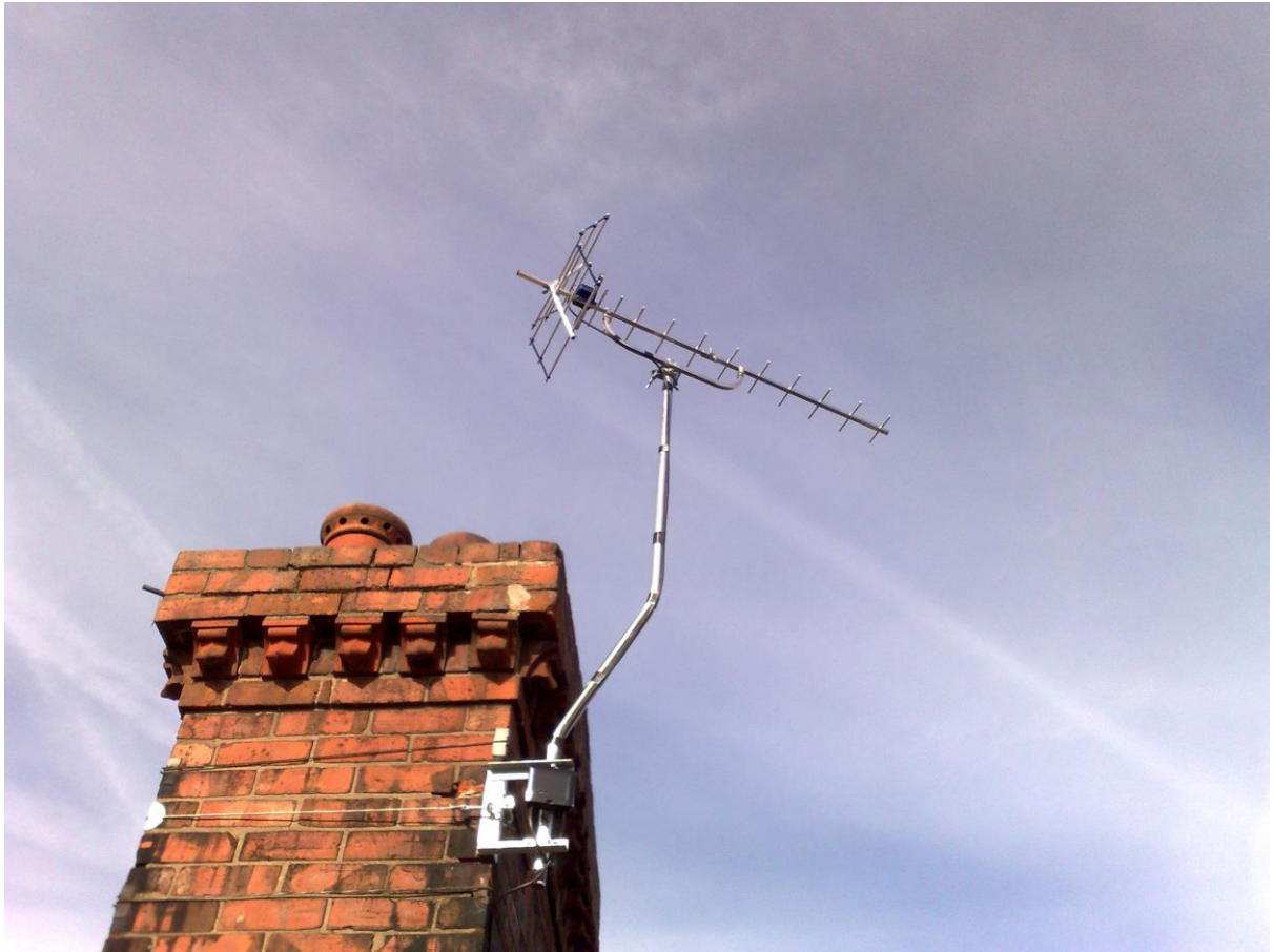
Example of TV aerial and fixings
