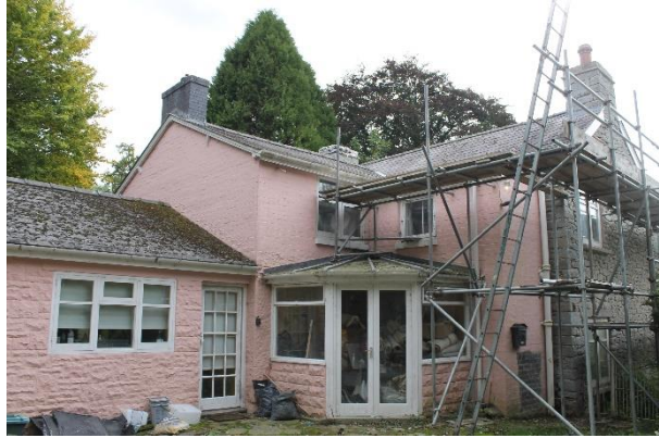
Plate 2: View of the house from the N showing kitchen to left of image
