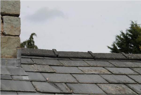
Plate 5: View of the roofline showing potential for bat access to ridge channel and chimney stonework
