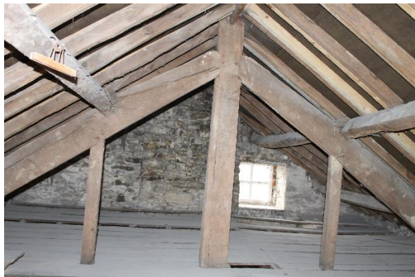
Plate 8: View of the main roof with 1F felt and existing light source
