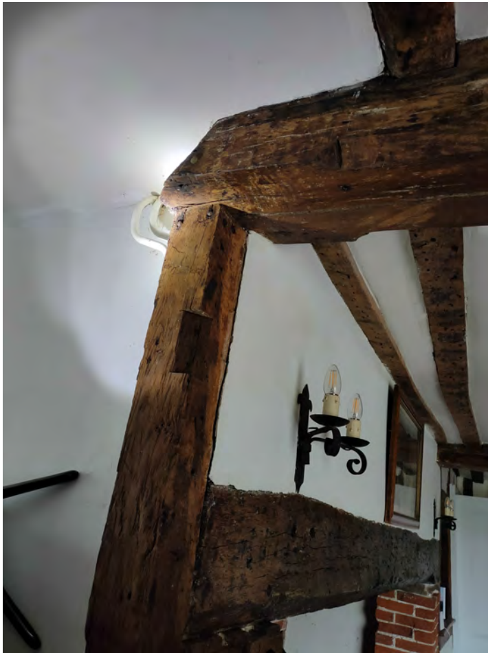
Fig 21 -South ceiling beam supported on stud bolted to S. side of inglenook- no hands tech!
