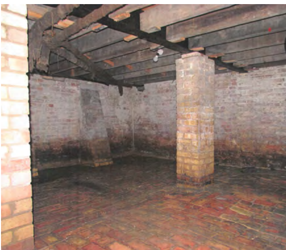
Fig 19: brick basement with later pier
