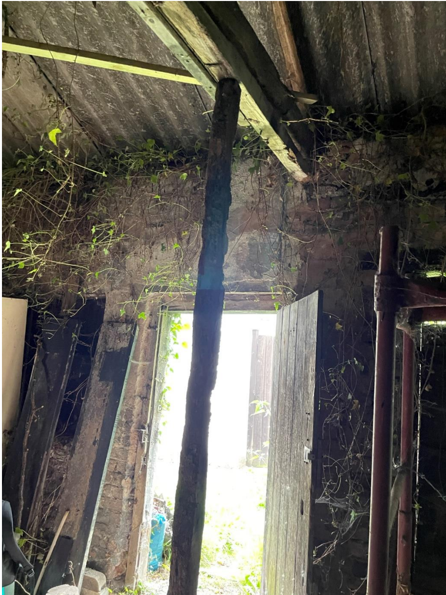
Photo 15. Interior side door entrance showing beam used to shore up the roof structure.
