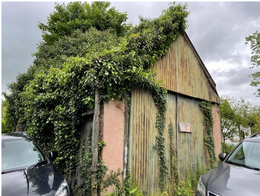
Photo 2. The northwest elevation showing extensive ivy growth
