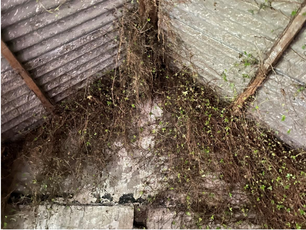
Photo 9. Interior showing ivy penetration and wooden beam roof structure
