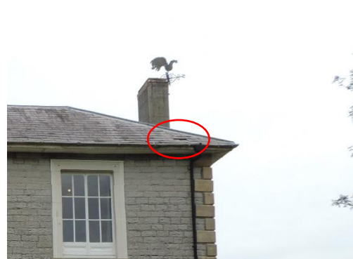
Plate 4: Example of Missing Tile
