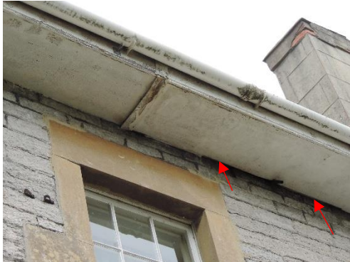
Plate 3: Example of Gaps Behind Soffit Box
