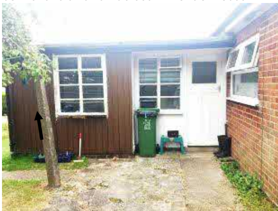
Photo 3. View north of rear single storey extension. Metal window frames. Flat roof in good condition and no gaps for bat or bird access.
