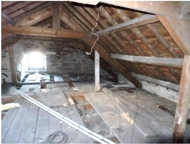
Photograph of the loft area showing wooden sarking (from 2011 report R Hadden)
