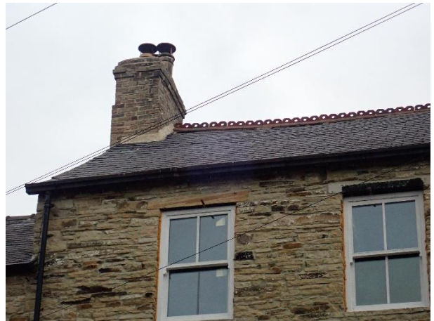
Possible crevices below the ridge tiles
