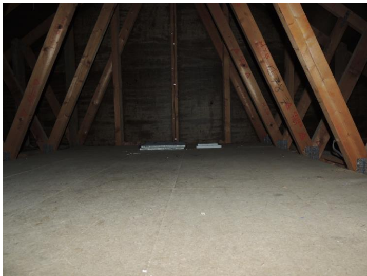
Photo 5: There was no evidence of bats on the floor of the loft
