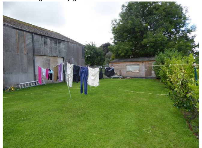
Northern asbestos clad elevation of the Dutch barn with surrounding amenity grassland / wooden garage in background and cherry laurel hedge north of the barn.
