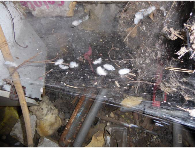
Pigeon feathers caught on cobwebs below wooden box in top NW corner of the barn.
