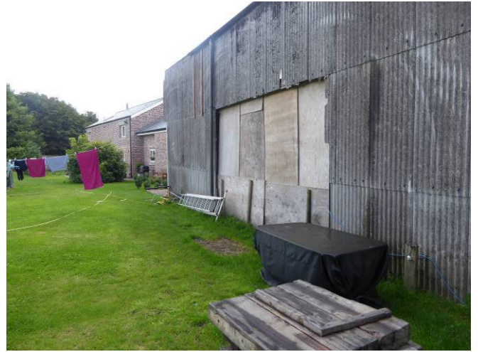
Northern asbestos clad elevation of the Dutch barn with surrounding amenity grassland.
