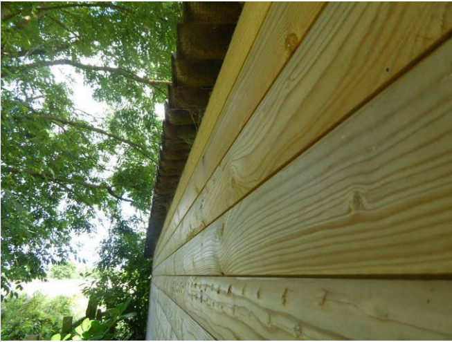
Wooden garage with corrugated roof on the sites western boundary, showing the western elevation.
