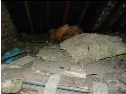
Photo 18. Floor conditions of large loft void
