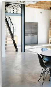
insert steel frame as new supports for timber truss/rafter roof as part of mezzanine deck frame
