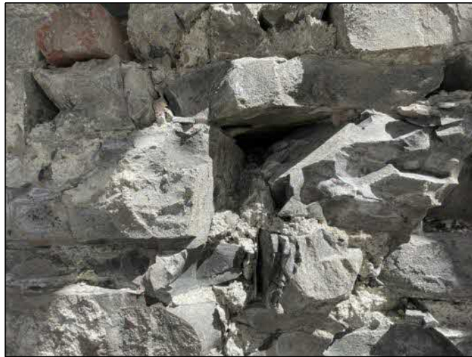
Plate 14. Example of gaps in stonework
