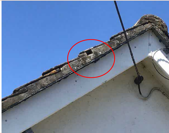
4. Gaps under tiles suitable for use by bats
