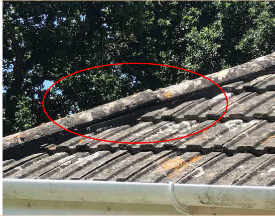
6. Gap under ridge tiles
