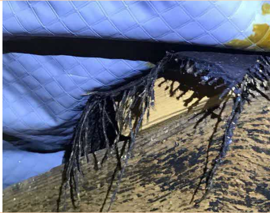
2. Gap around roof timber and gap in membrane
