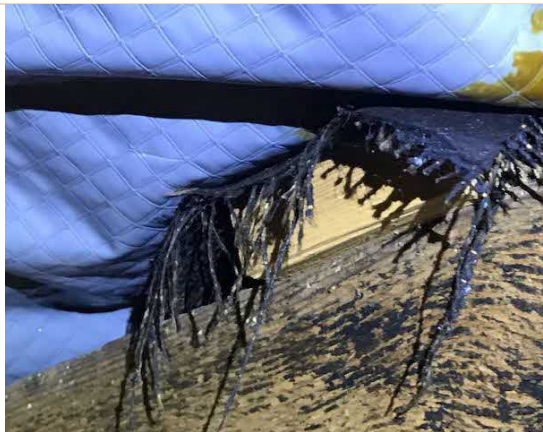
Gap around roof timber and gap in membrane
