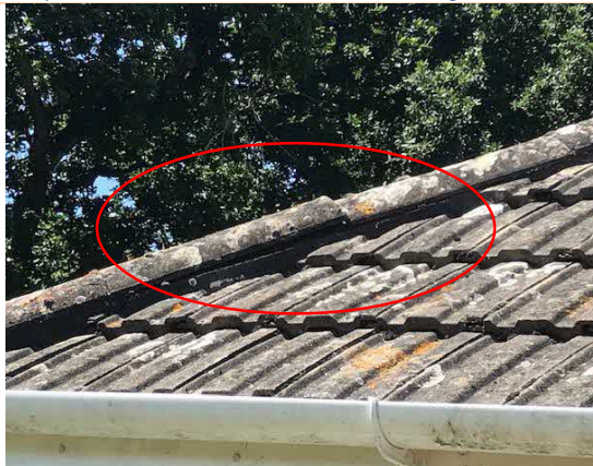
Gap under ridge tiles
