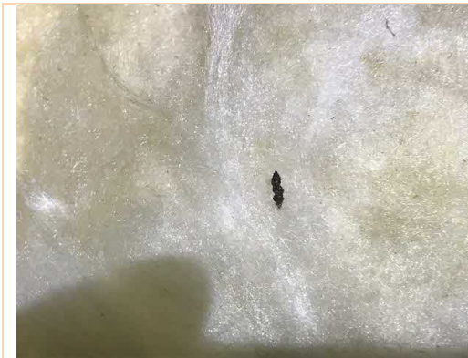
Bat dropping found on loft floor
