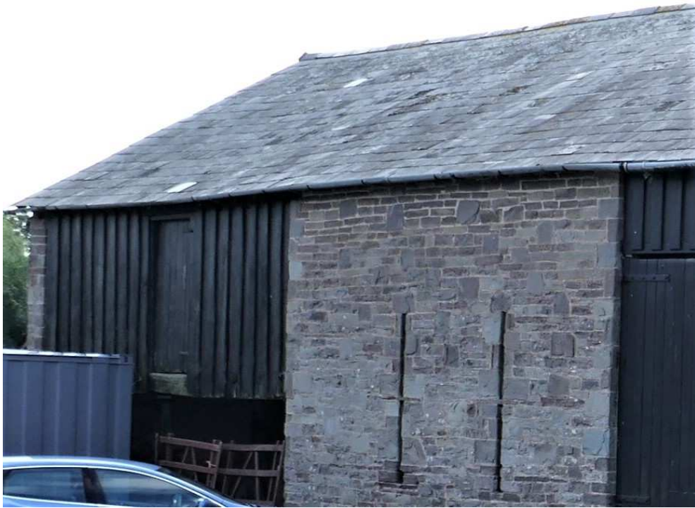
6. The open fronted cart shed and the wall of the threshing barn with extensive rebuilding above the vent slits.
