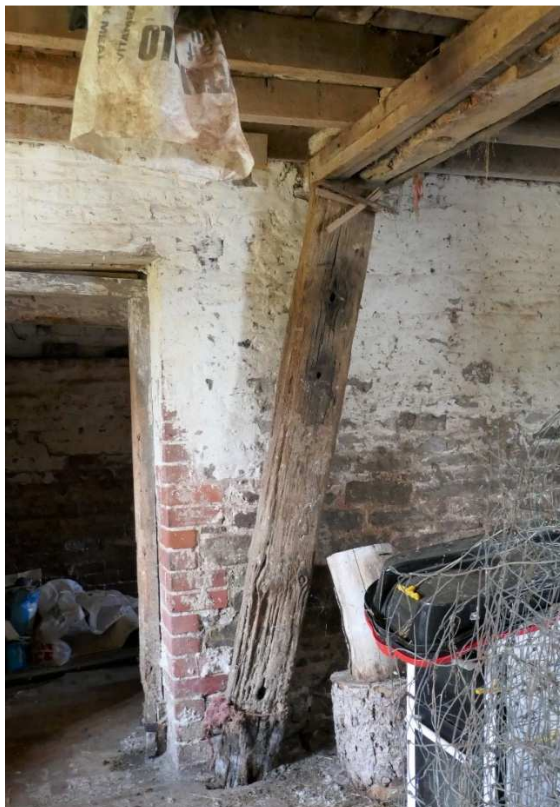
6. Defective timberwork in the Cowhouse
