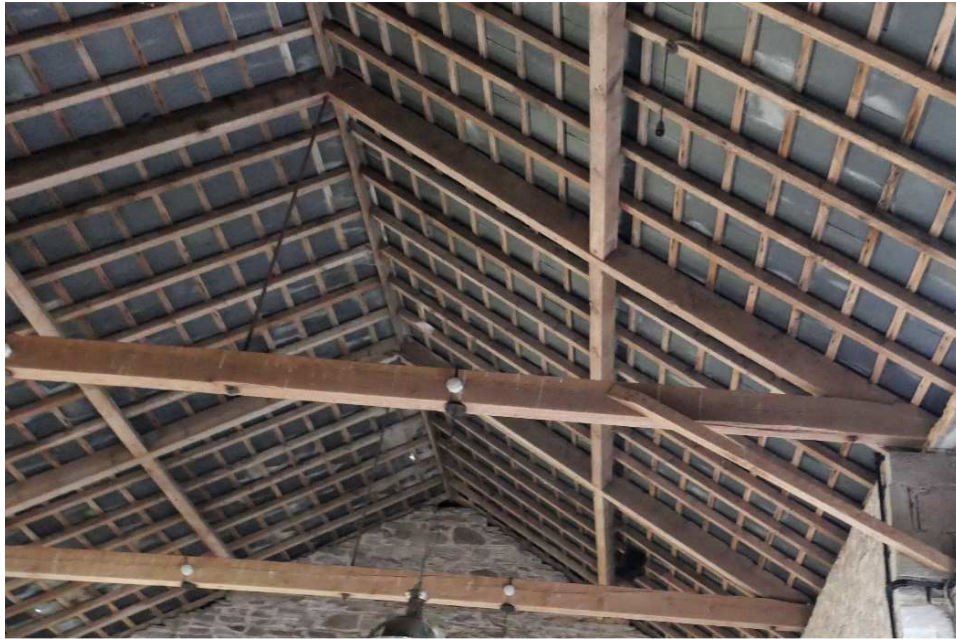
9. The undersized rafters and trusses in the Threshing Barn
