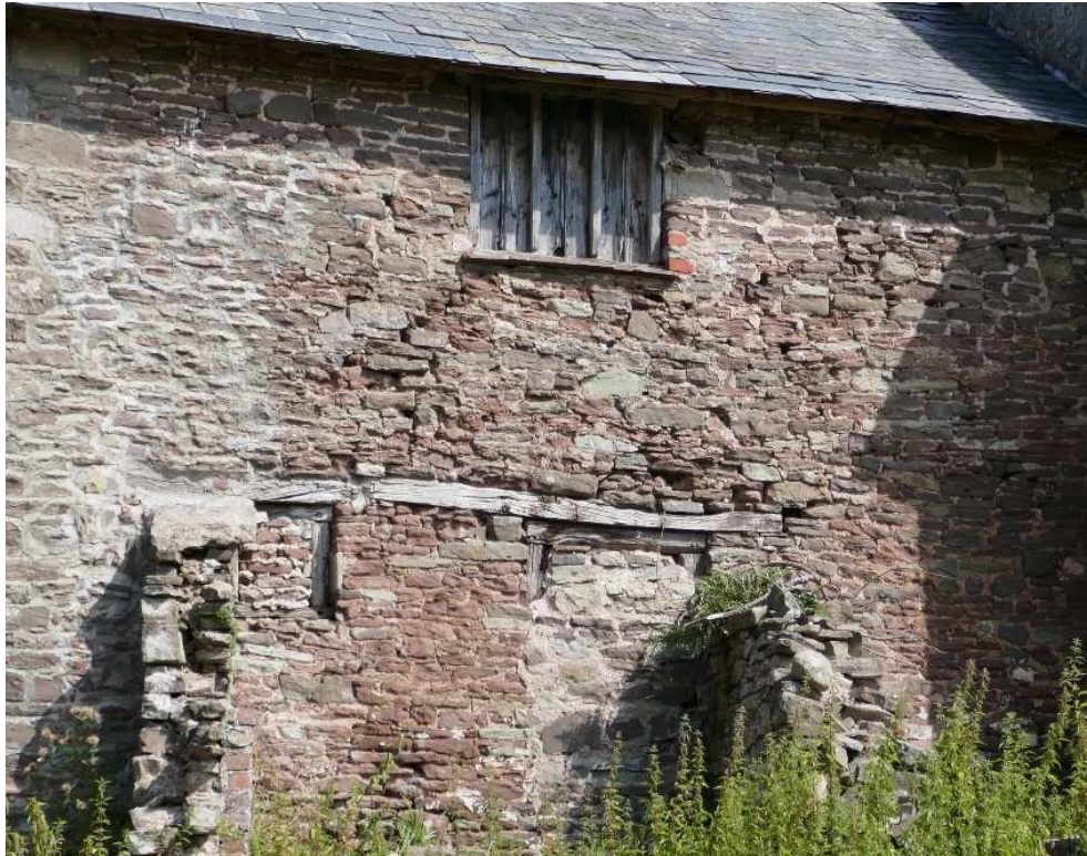
3. The south side of the Cider House requires rebuilding of the outer skin of stonework
