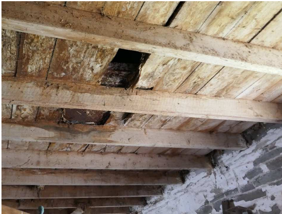
14. Damp affecting floorboards and joists in the Cow house
