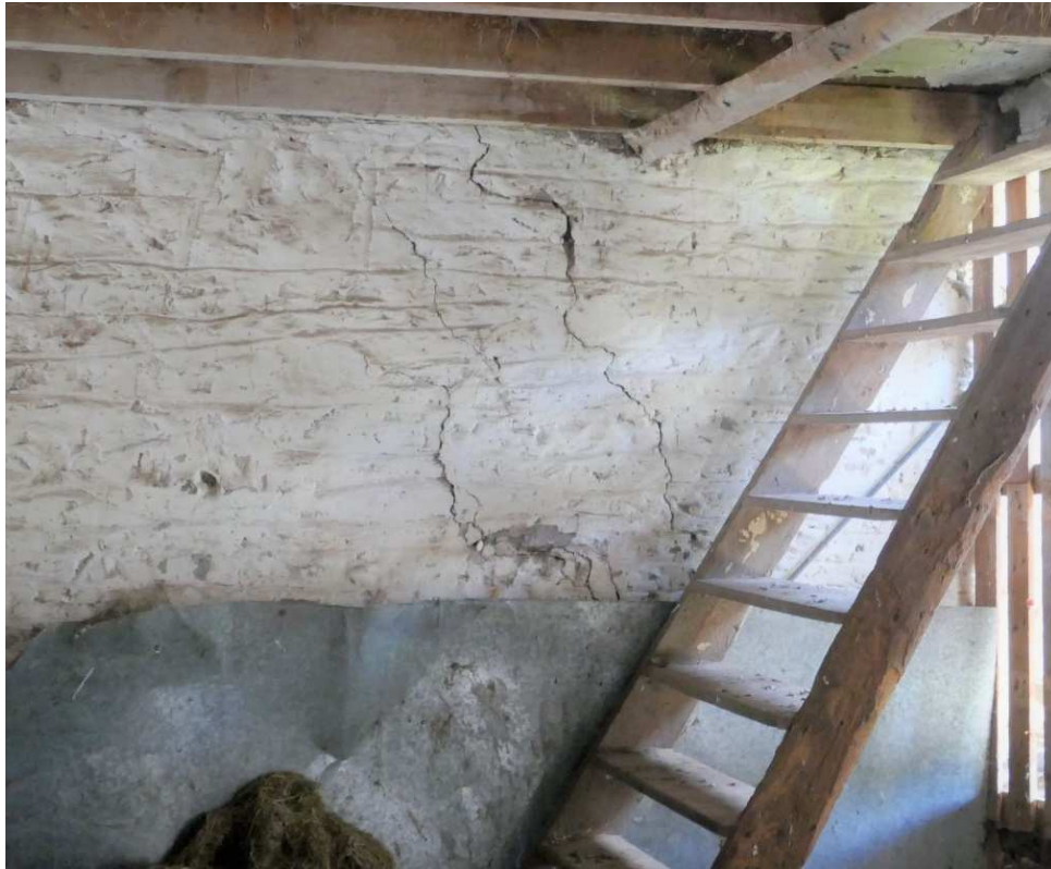
5. The same crack on the Cowhouse side
