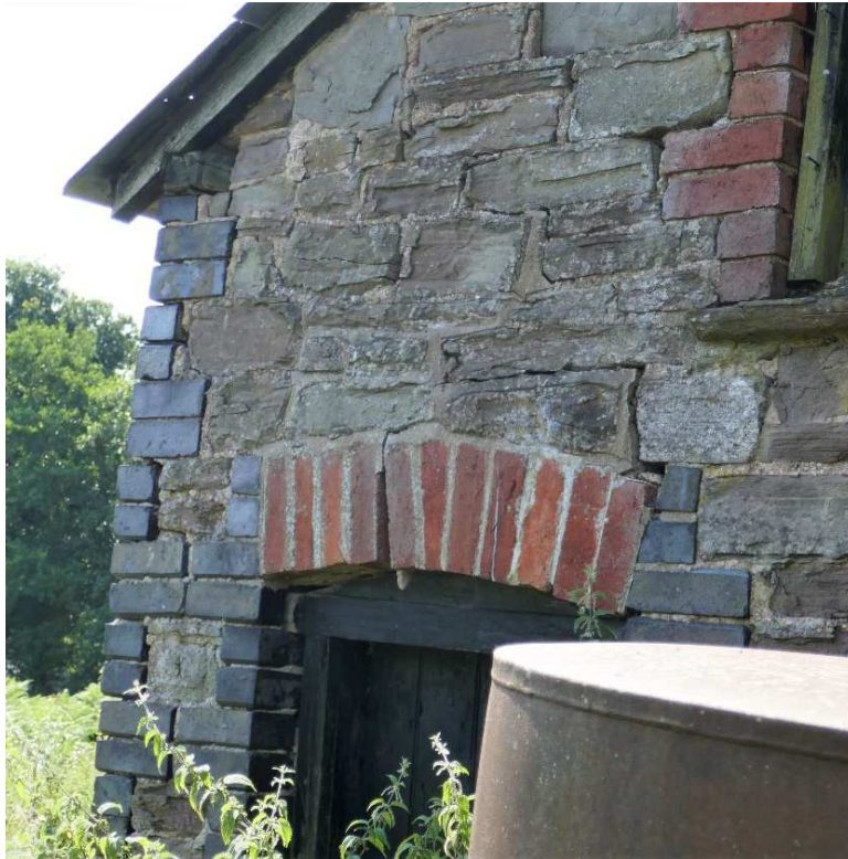
1. The doorway and quoins of the Fowl House require rebuilding
