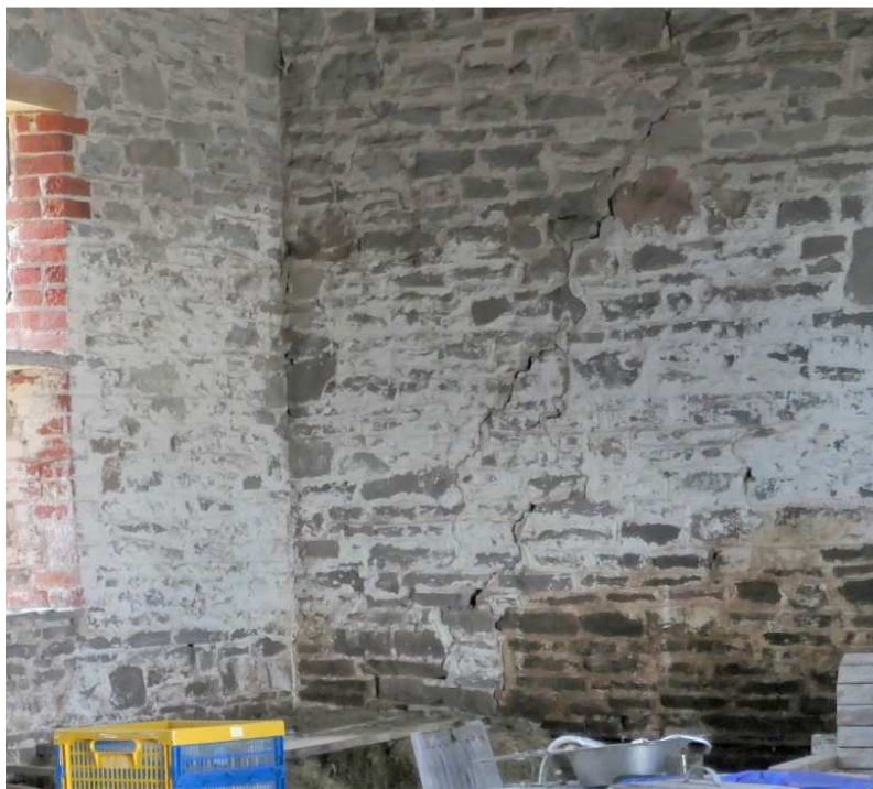
4. The internal cracking in the Threshing Barn
