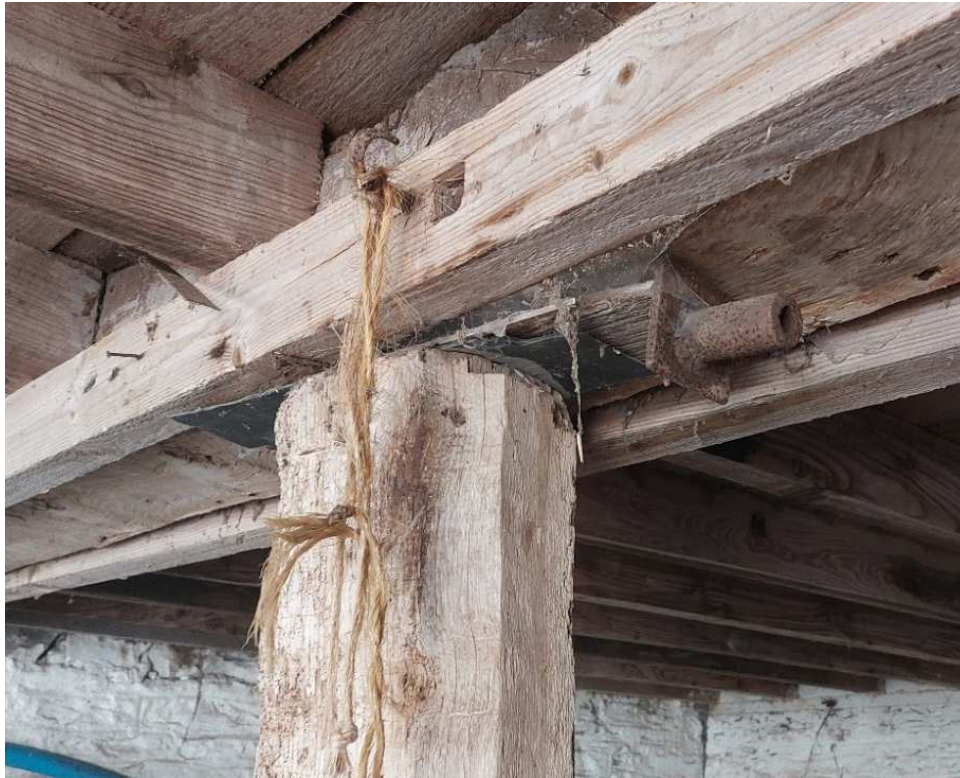
7. The beam across the cart shed with nailed on bearers for the floor joists on each side. Note the steel packer.
