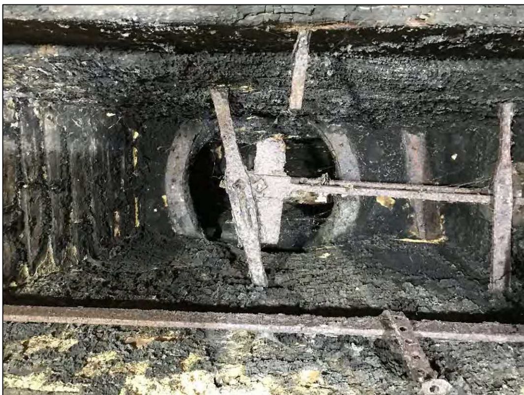
34. Outbuilding 1: chimney breast interior. Smoke jack mechanism (c. 18 th century)
