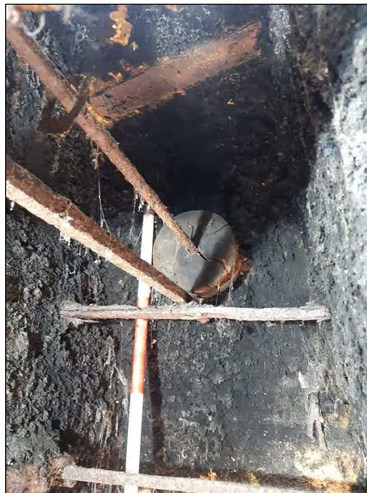
33. Outbuilding 1: chimney breast interior. Smoke jack mechanism (c. 18 th century)
