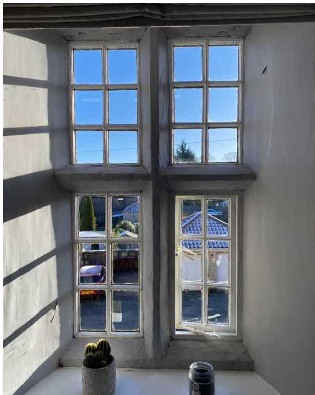
Above is inside view of window No 3. Only bottom right part opens on hinges. Window is 82cms x 148cms
