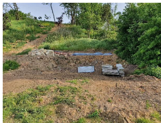
Terraces and materials stockages areas to be converted into the adopted landscape plan
