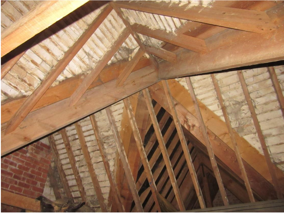
Figure 29: The original roof structure at the junction with one of the extended south-east gables.
