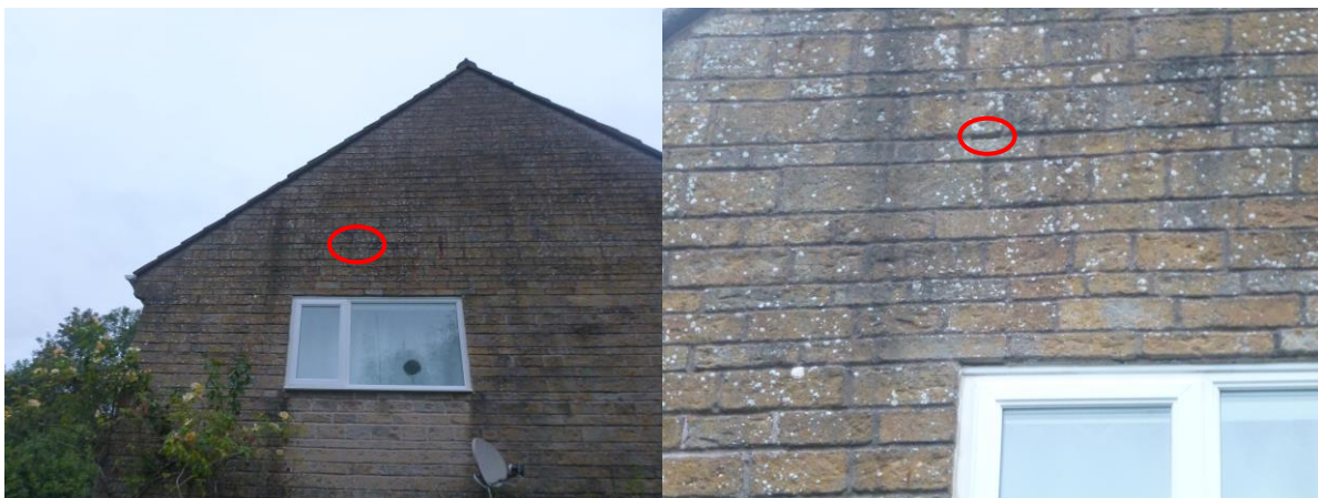
Fig 8: Crevice in the brickwork on the southern aspect of Old Mill where five soprano pipistrelle bats were recorded roosting during a re-entry survey carried out on 30 th August 2021.
