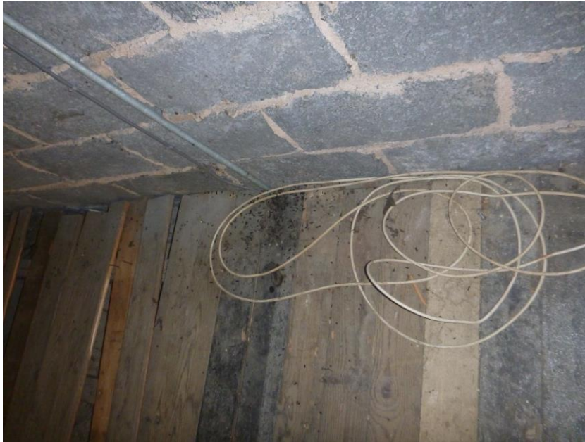
Fig 5: An accumulation of serotine droppings against the northern gable end wall of the loft space.
