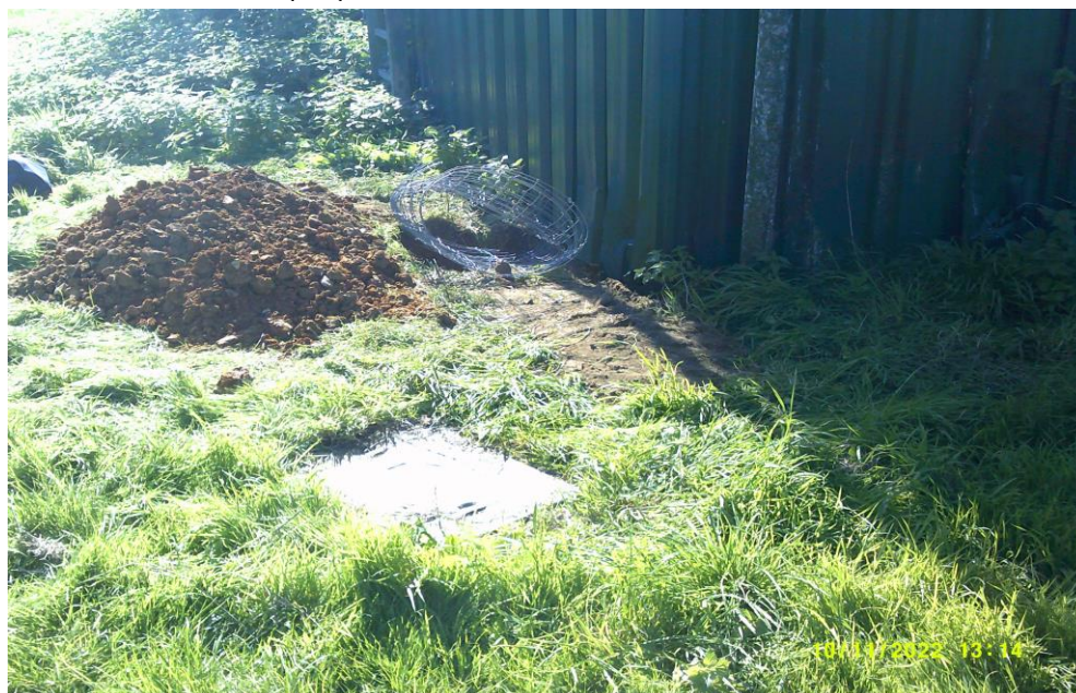
Frame No: 06 Location: The Cold Store, Butlers Farm, Horseshoes Lane, Maidstone, Kent ME17 3JY Description: A drain manhole cover adjacent to the rear right hand corner of the building and near the trial pit in photo 04 Date: 11/10/22
