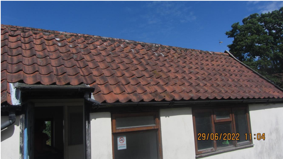
Photo 1: View of southern aspect Building 1 exterior, showing pantile roof which in areas has lifted
