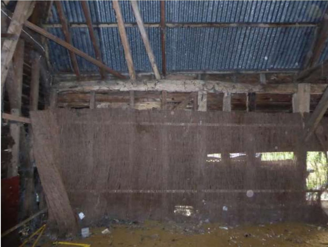
Photo 19: The western part of the internal north elevation of the barn (partially obscured).
