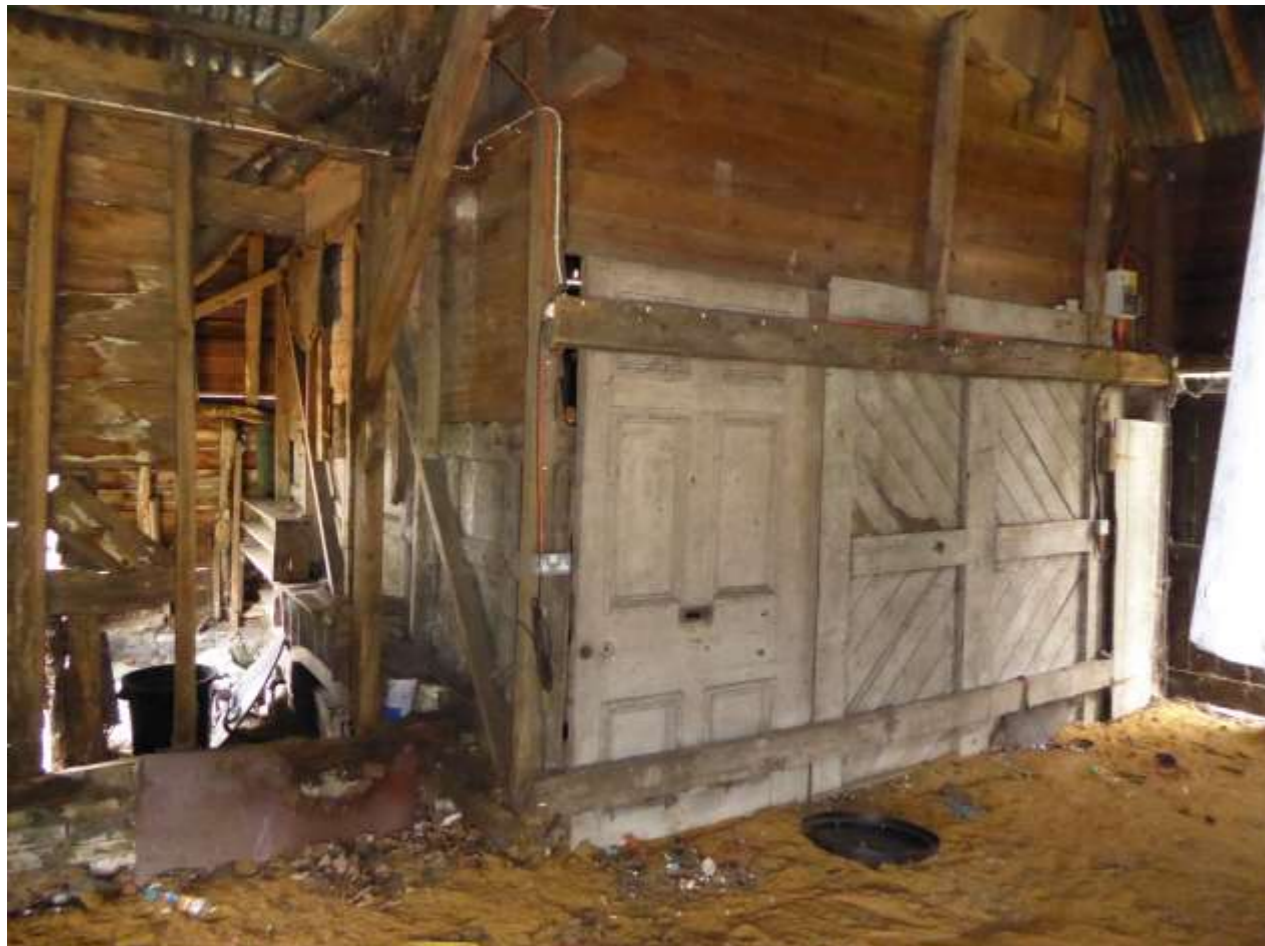
Photo 32: The internal south elevation of the northern part of the barn, looking towards the southern part.
