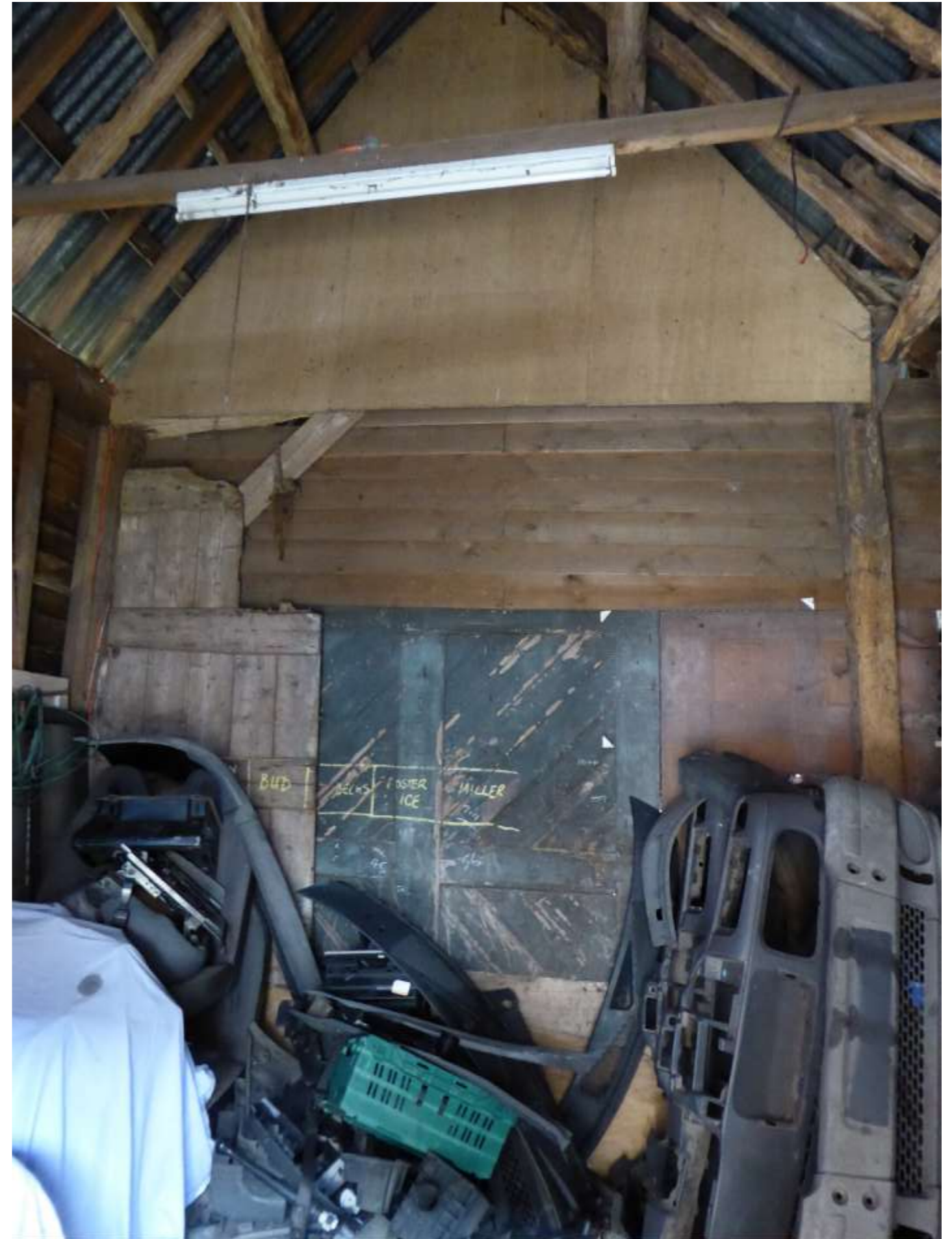
Photo 24: The internal 'partition' between the northern part of the barn and the southern part, from the south.
