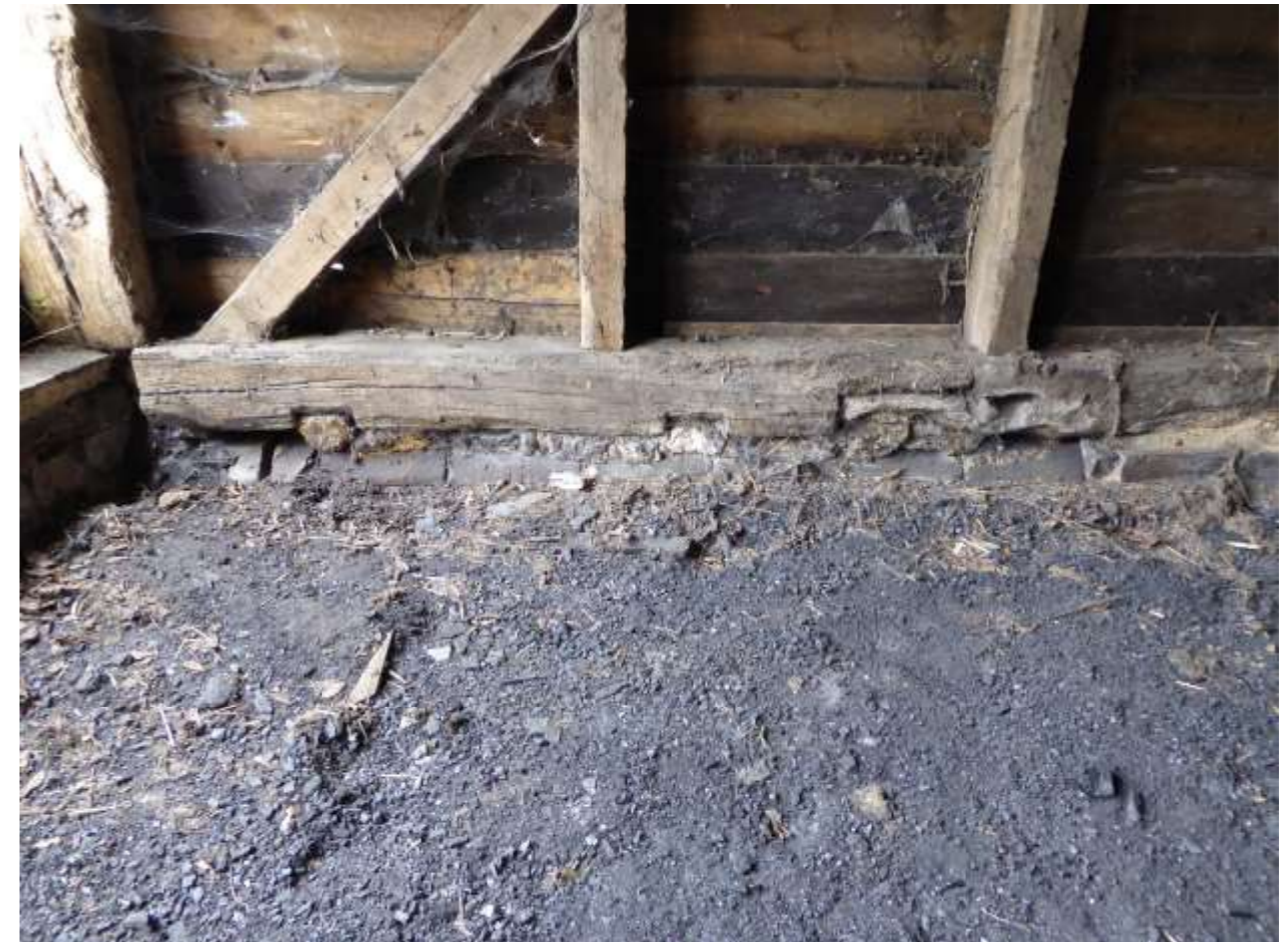
Photo 22: Detail of the sole plate in the internal east elevation of the barn.
