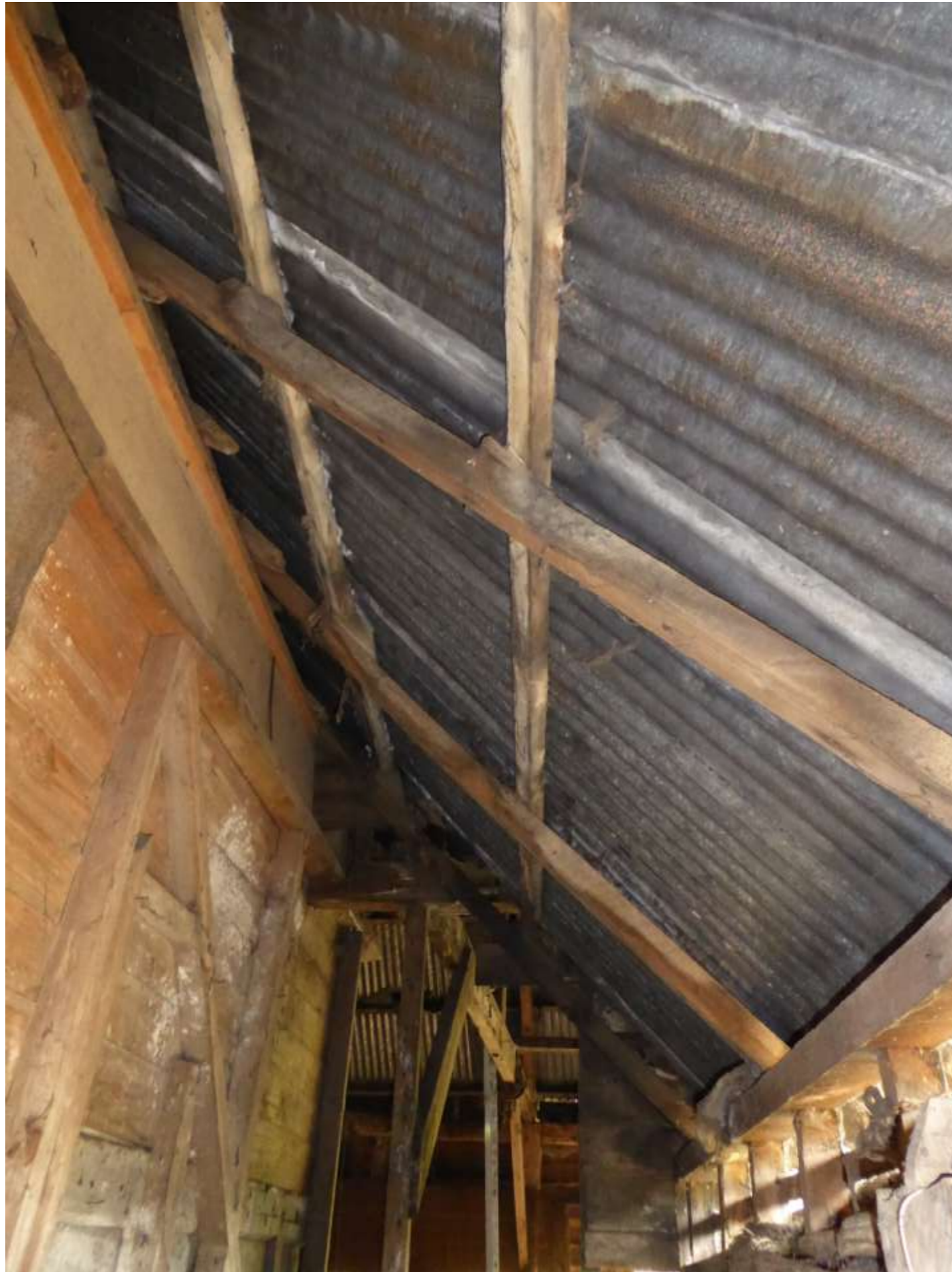
Photo 37: The roof structure (looking north) of the eastern room with catslide roof.
