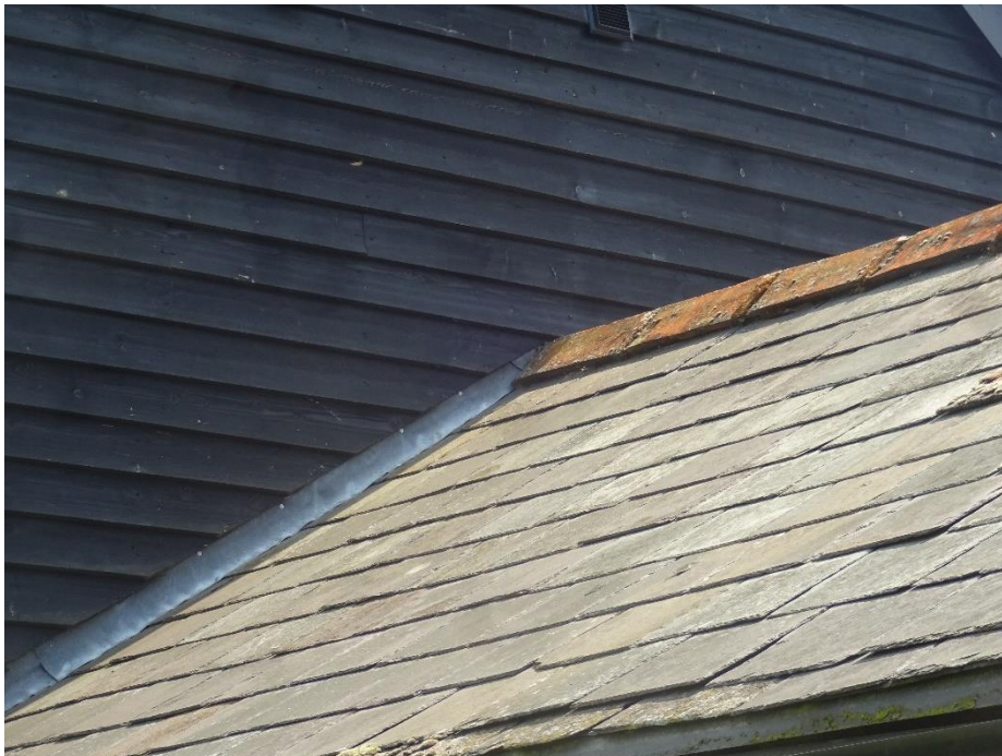
Photograph 10: View of join between adjacent building and outbuilding above location bat droppings observed. 7 th May 2020.
