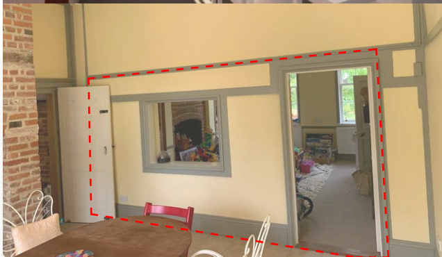
Opening up between former kitchen room and drawing room. Positioning the kitchen / diner on this side of the house will reinstate the original function to this space.
