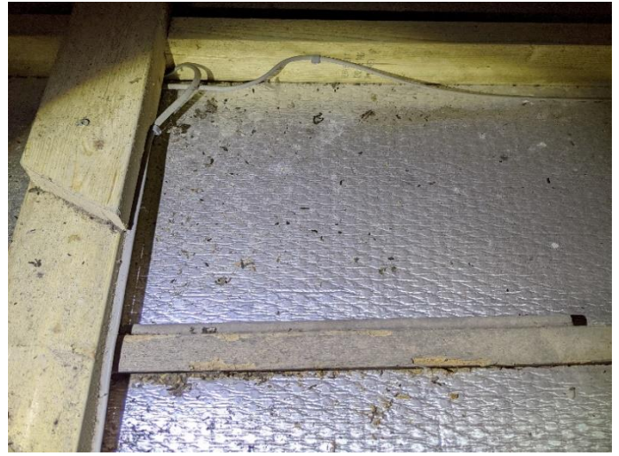
Photo 20 Scattering of BLE and pipistrelle droppings on the floor in the cottage loft
