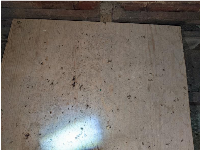
Photo 19 BLE droppings on the floor beneath the ridge in The Grange northern loft
