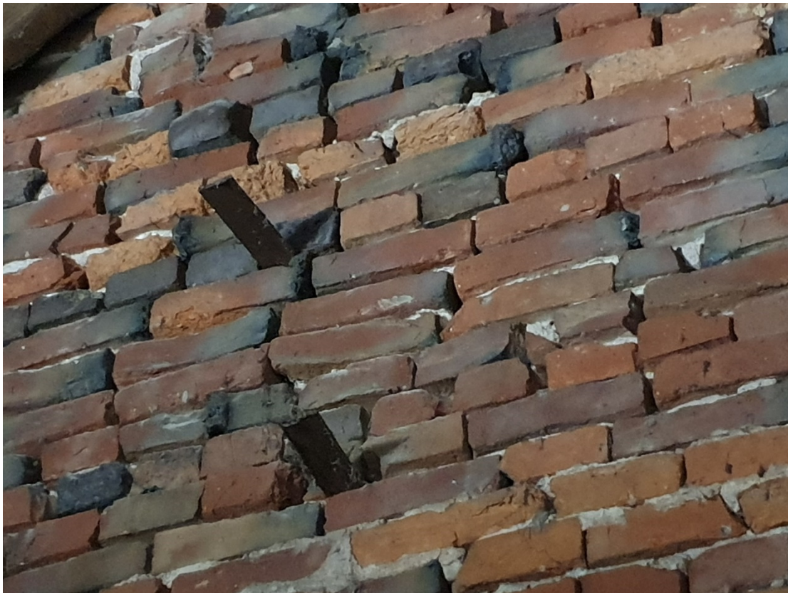
Photograph No. 12 – Poor bonding and missing mortar to the internal face of the gable wall to building no. 3
