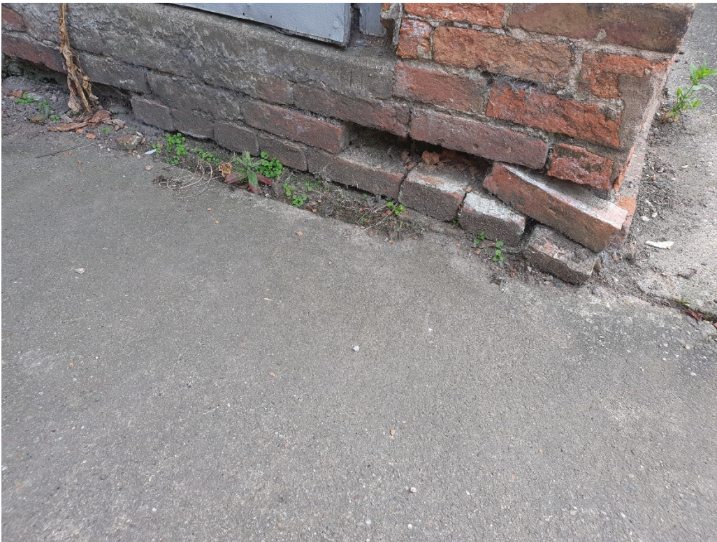
Photograph No. 17 – Missing and loose low level brickwork to the NW corner of building no. 4
