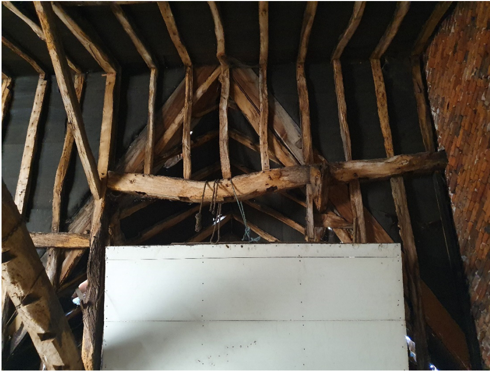
Photograph No. 9 – Irregular roof timbers to building no. 3
