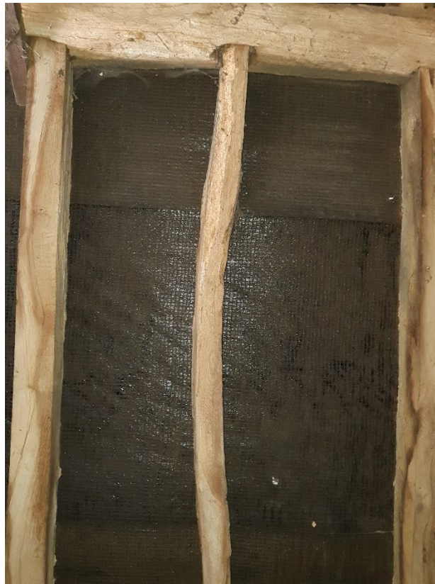
Photograph No. 10 – Undersized rafter to building no. 3
