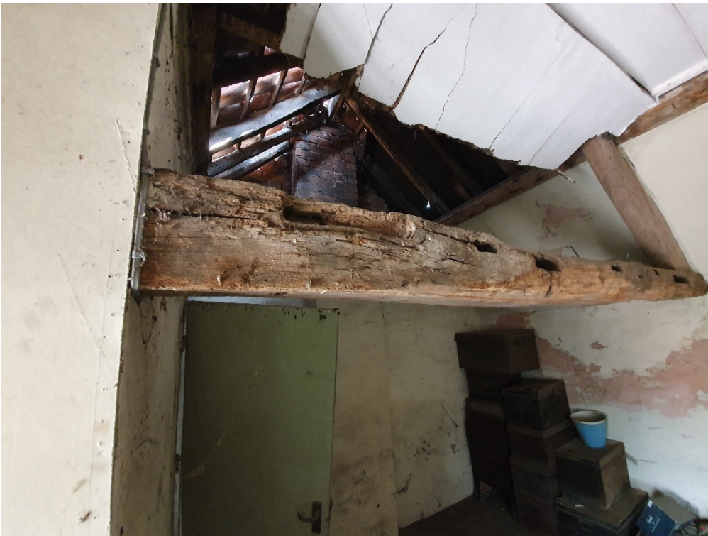
Photograph No. 19 – Defective roof frame to building no. 5
