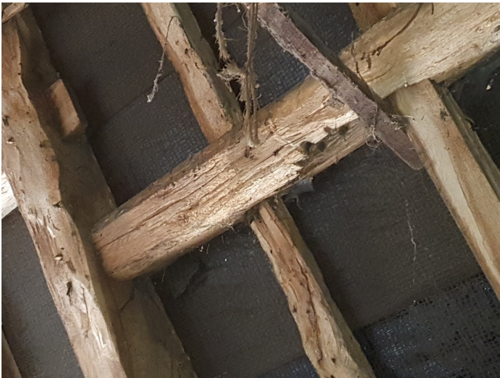
Photograph No 8 – Defective roof timbers to building no. 3
