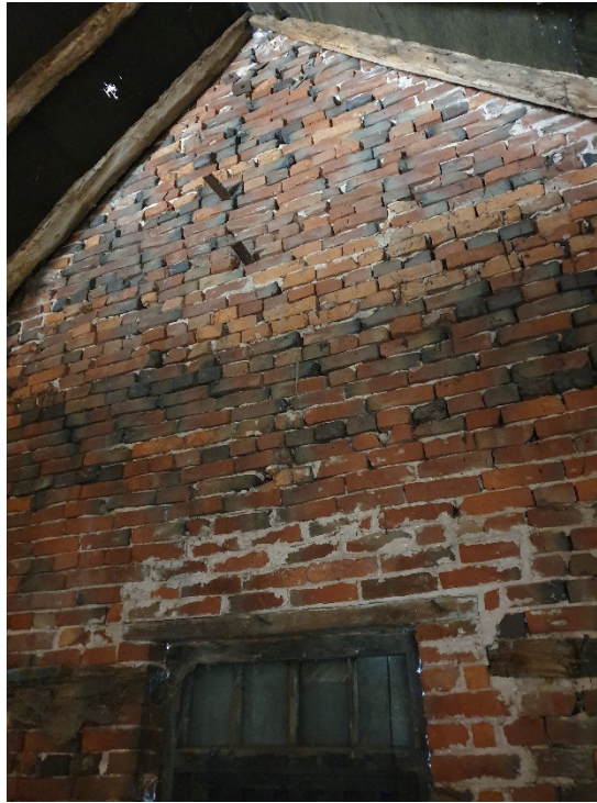
Photograph No. 11 – Internal view of high level masonry to the gable wall of building no. 3
