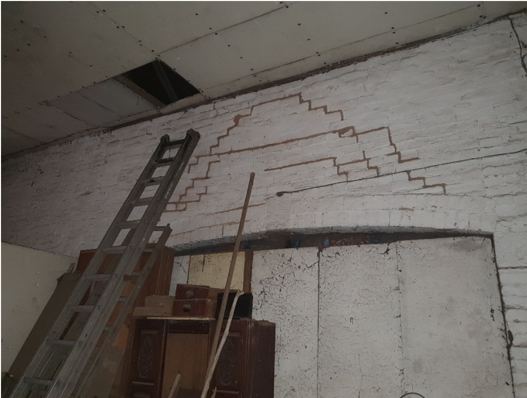
Photograph No.15 – Masonry movement and cracking over shallow arched opening to building no. 4
