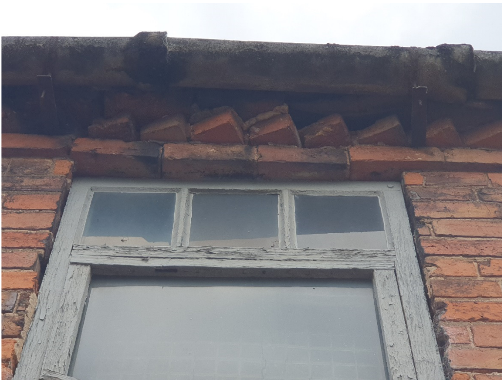
Photograph No. 18 – Loose and deflected brickwork over opening to building no. 4
