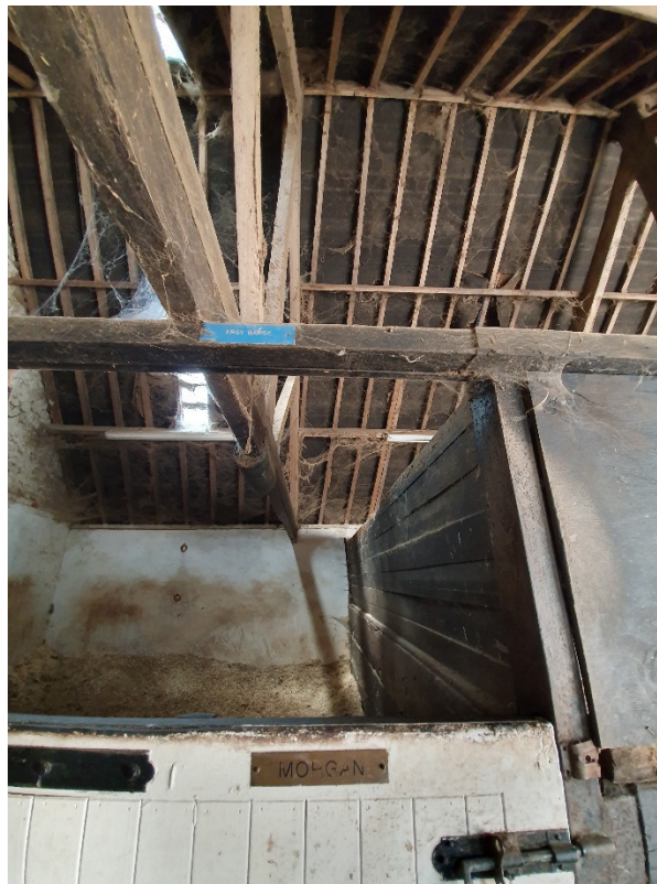
Photograph No. 2 – Timber truss to building no. 1 out of plumb
