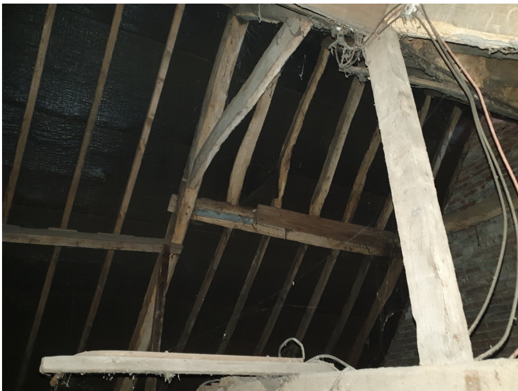
Photograph 14 – Bowed member to principal timber roof frame to building no. 4
