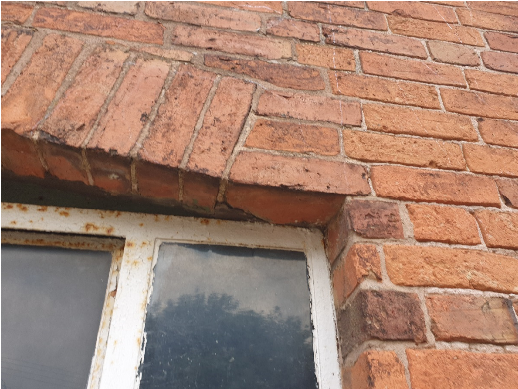
Photograph No. 16 – Defective arch springing point to opening in building no. 4
