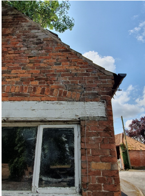
Photograph No. 5 – Cracking to the North gable wall of building no. 1
