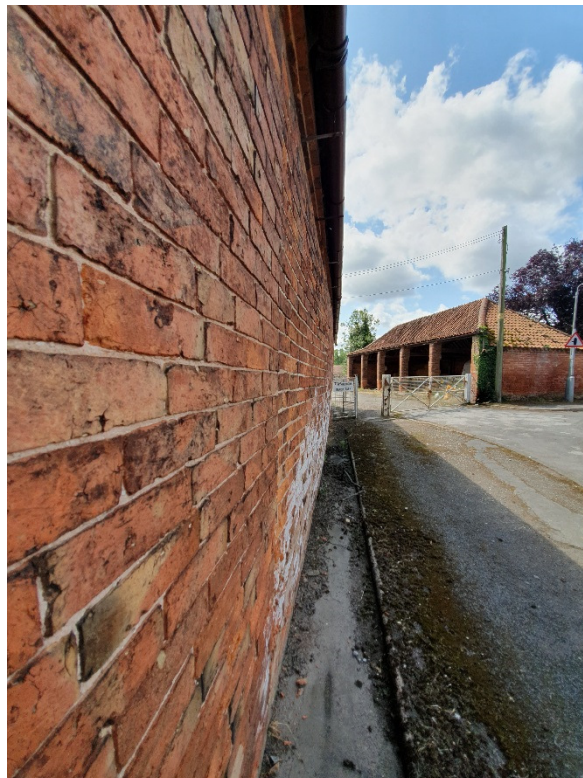
Photograph No. 6 – Outward bulge to the West wall of building No. 1
