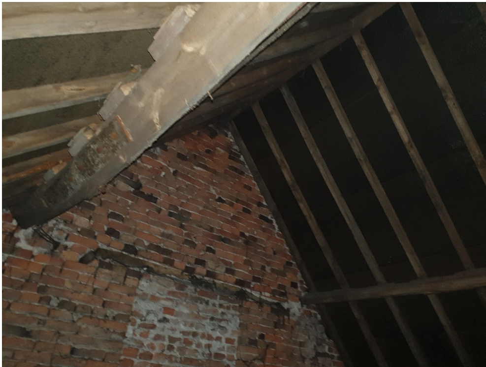
Photograph No. 13 – Deflected and split purlin to building no. 4
