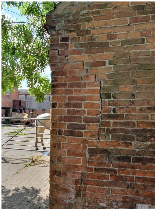
Photograph No. 4 – Cracking to the North gable wall of building no. 1
