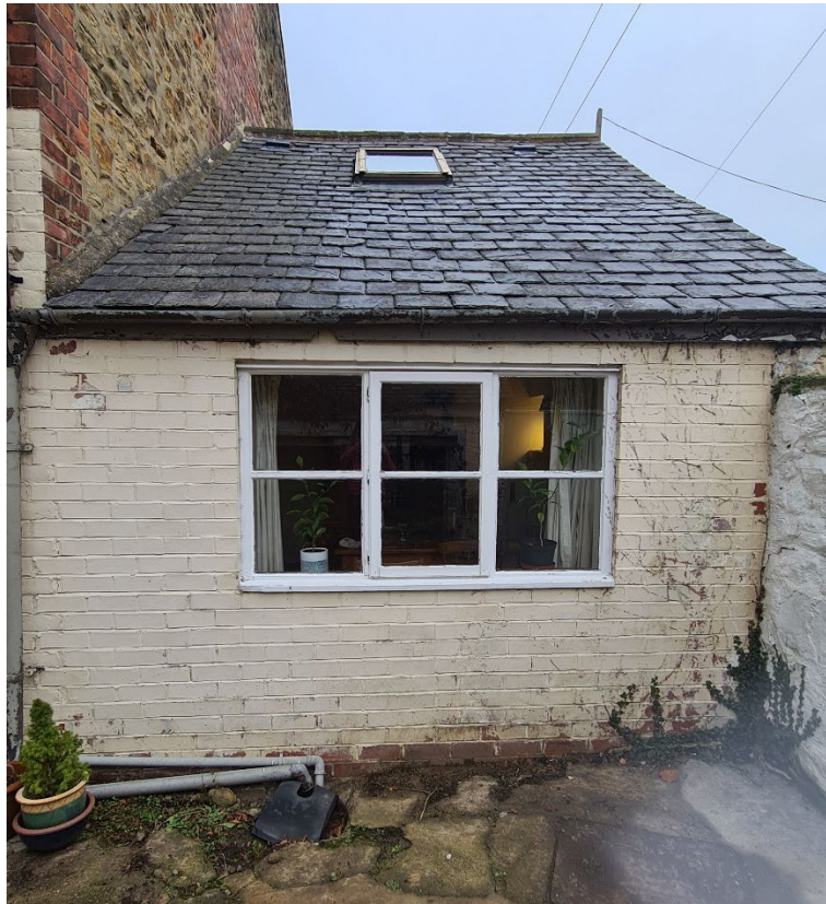
Figure 3.1: Single-storey rear of the house with existing window (to be converted into sliding doors accessing the yard) and 1no. rooflight (to be replaced with 2no. rooflights)
