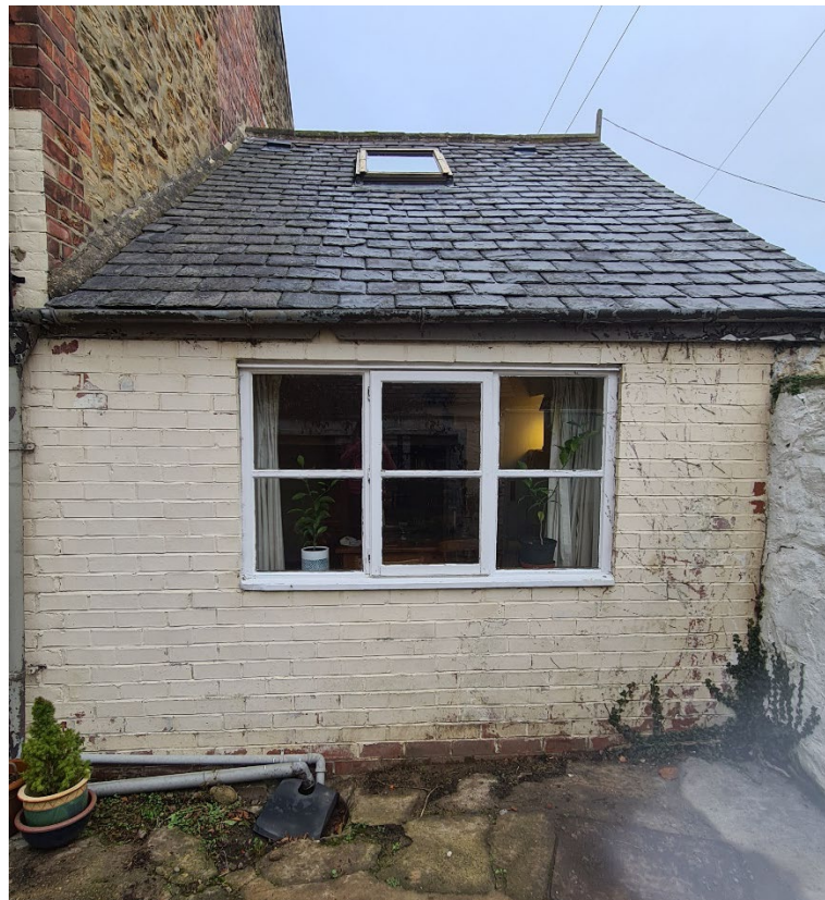
Figure 2: Single-storey rear of the house with existing window (to be converted into sliding doors accessing the yard) and 1no. rooflight (to be replaced with 2no. rooflights)
