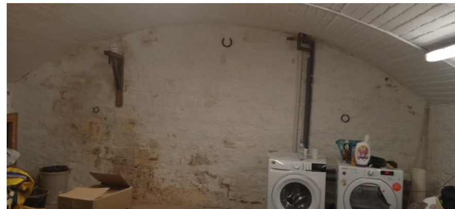
Inside the garage space showing brick vaulted ceiling at the east (underground) wall
