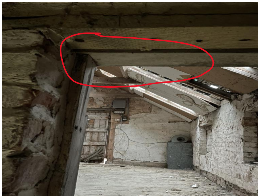
Photograph 21: Gap in timber lintels above doorway of upper floor of building 3 – transient roost site
