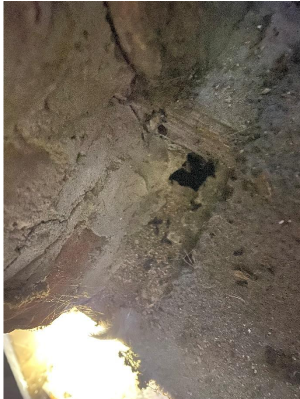
Photograph 20: Bat droppings beneath door way (below lintel niche) into upper floor of outbuilding 3
