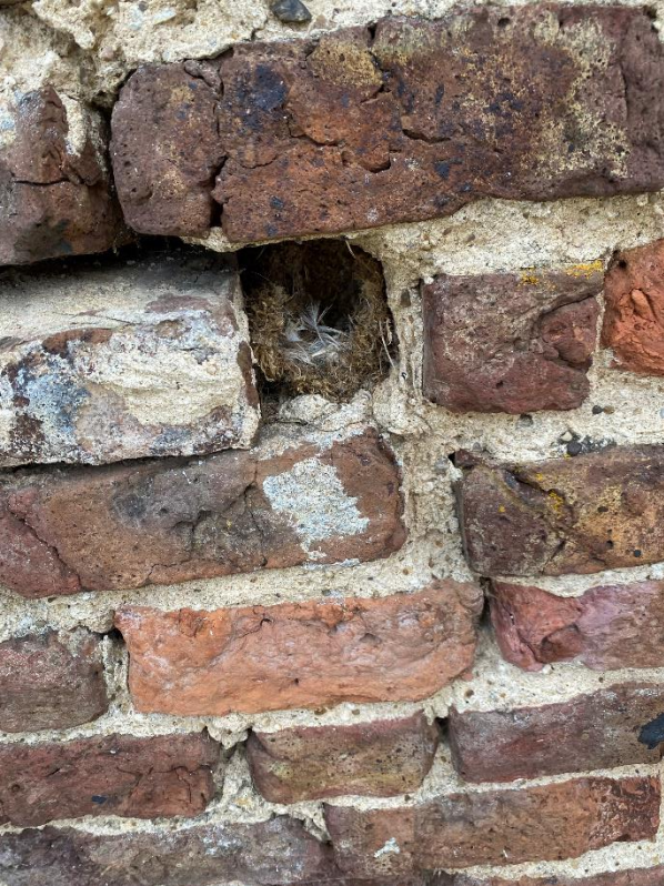
Photograph 24: Disused nest on the western elevation of outbuilding 4
